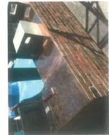
Copper flashing at capping
