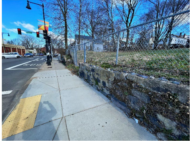
Photo 2: Retaining wall on the southwest side of the Property along Washington Street.
