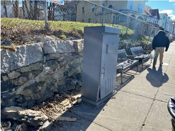
Photo 3: Pad mounted transformer on the sidewalk adjacent to the Property.
