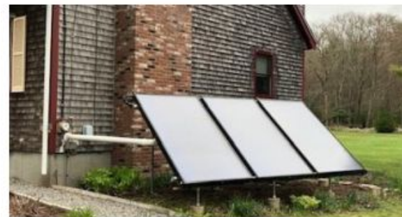
Solar hot water collectors installed on the ground.
