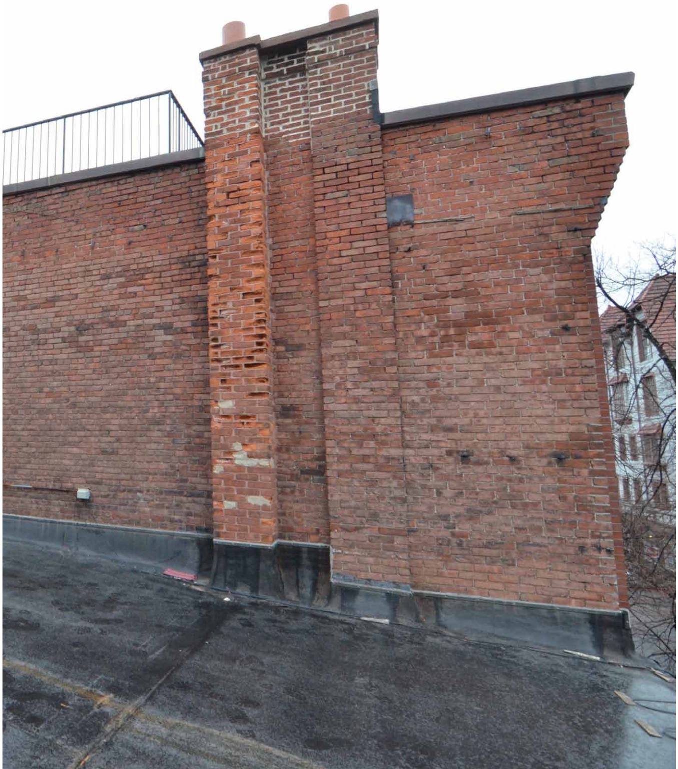
④ Existing chimney adjacent to 71 Chestnut Street to be re-built. Brick and mortar to match existing.
