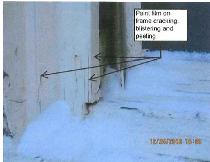
Frame Paint Failure
