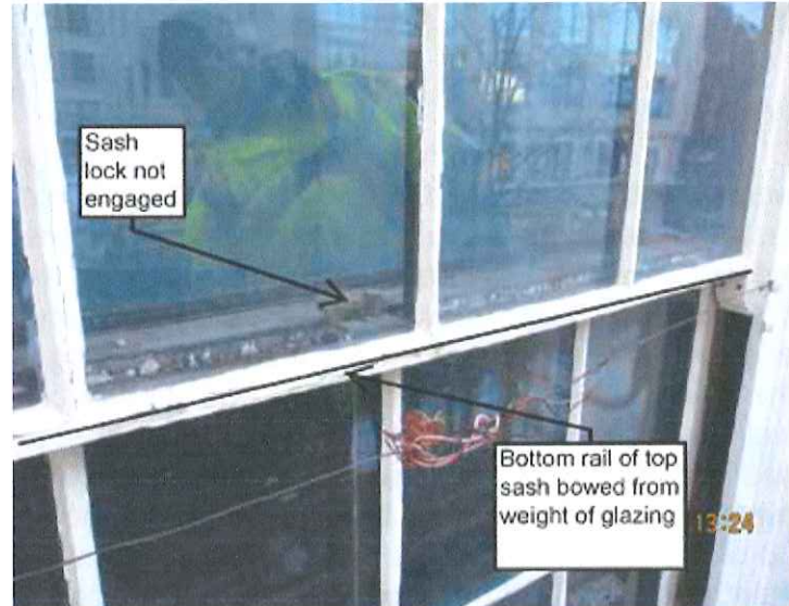
Bottom Rail of Top Sash Bowed
