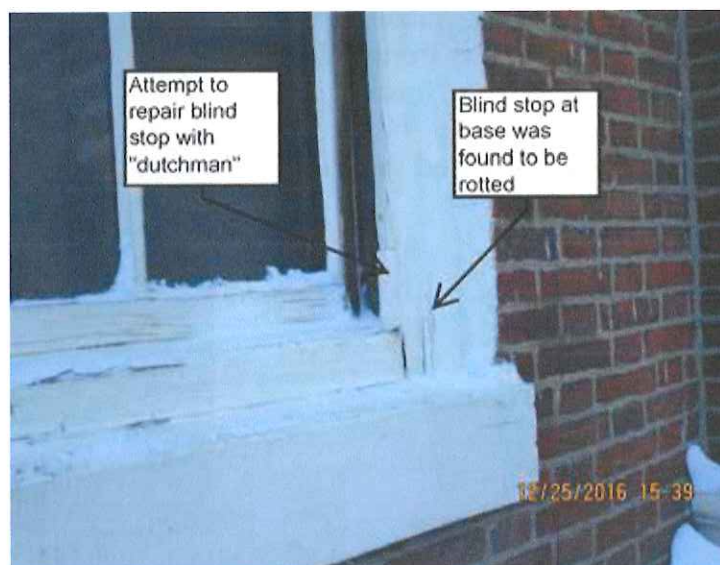
Blind Stop at Base Rotted
