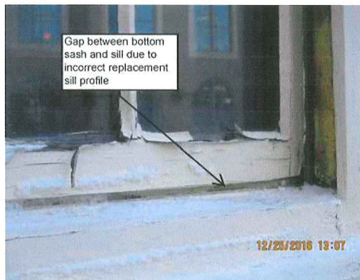
Bottom Rail of Lower Sash not closing tightly against sill
