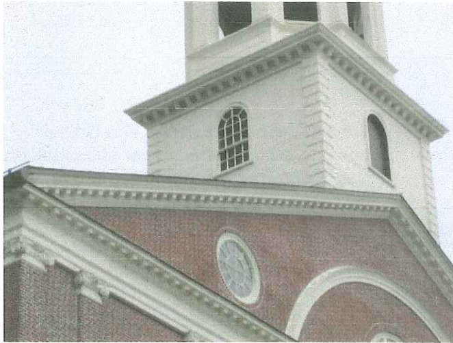
The condition of the paint coatings of the Faneuil Hall Bell tower in 2015
