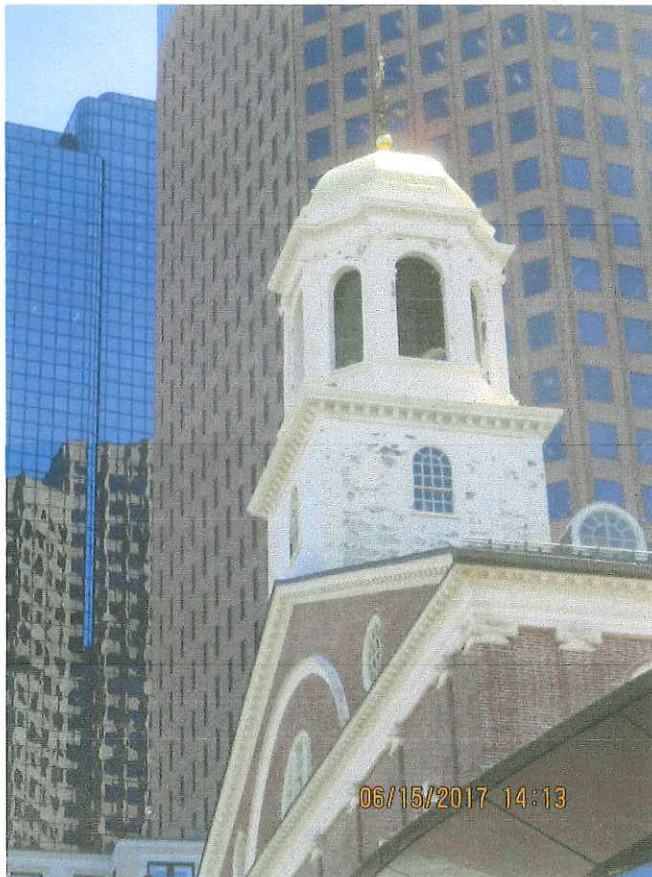
The condition of the paint coatings of the Faneuil Hall Bell Tower in 2017. The extensive failure of the paint coatings is the result of excessive re-coatings of the Bell Tower which has caused the paint film to finally pull away from the substrate due to excessive weight of the coatings.
