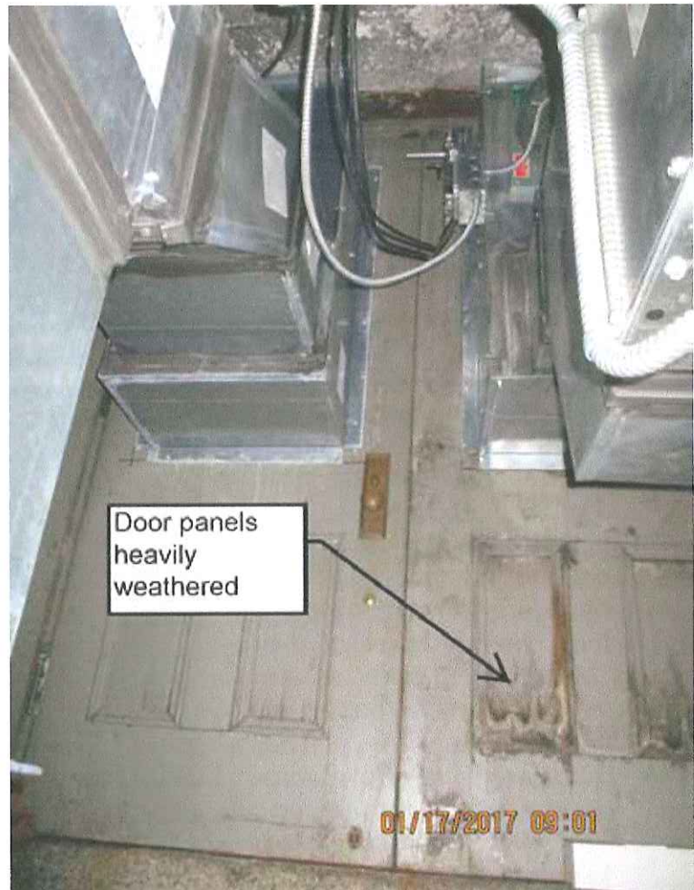
Basement Door Inoperable due to HVAC Ductwork
