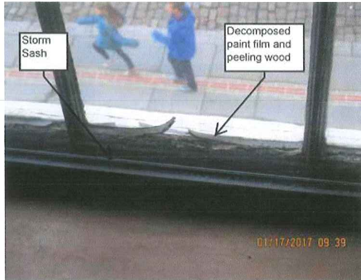
Major Deterioration of Bottom Rail of Sash at the Interior
