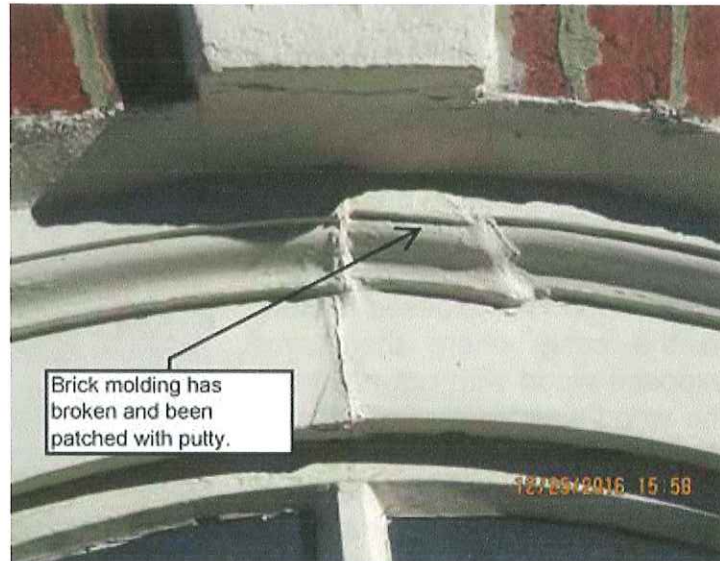
Brick Molding Broken
