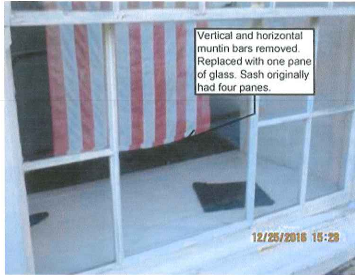
Cracked or Incorrect Glazing
