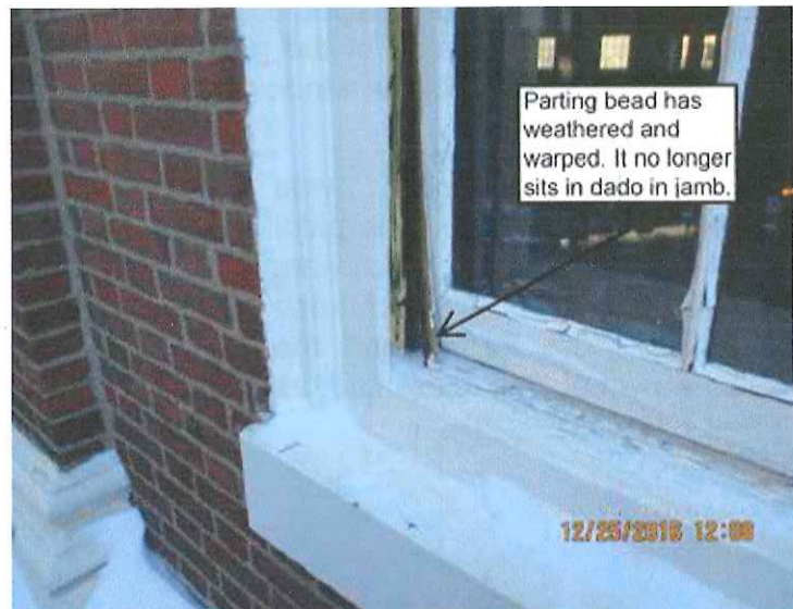
Parting Bead Displaced
