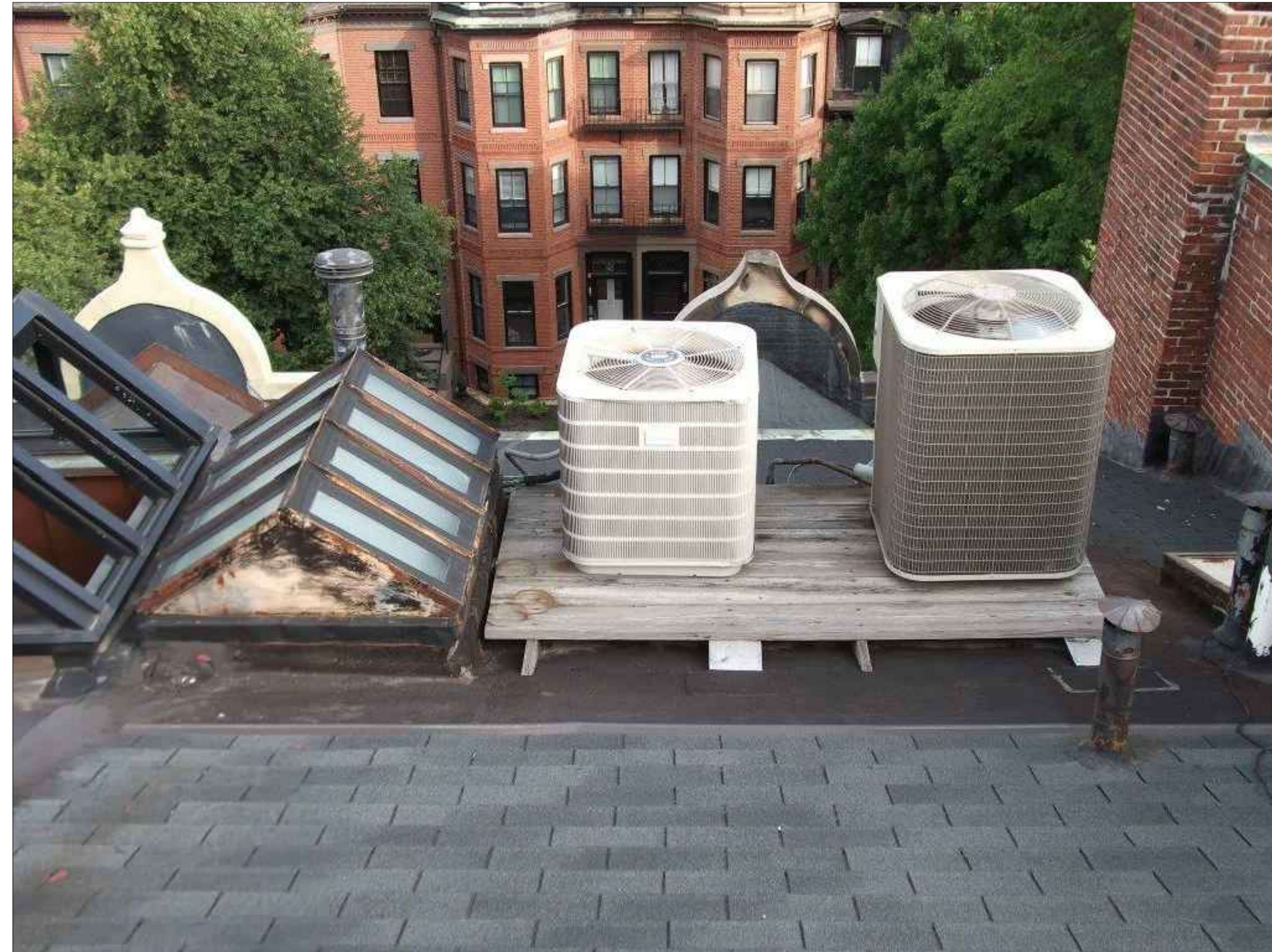
2 CONDENSOR (VIEW TOWARDS STREET)
