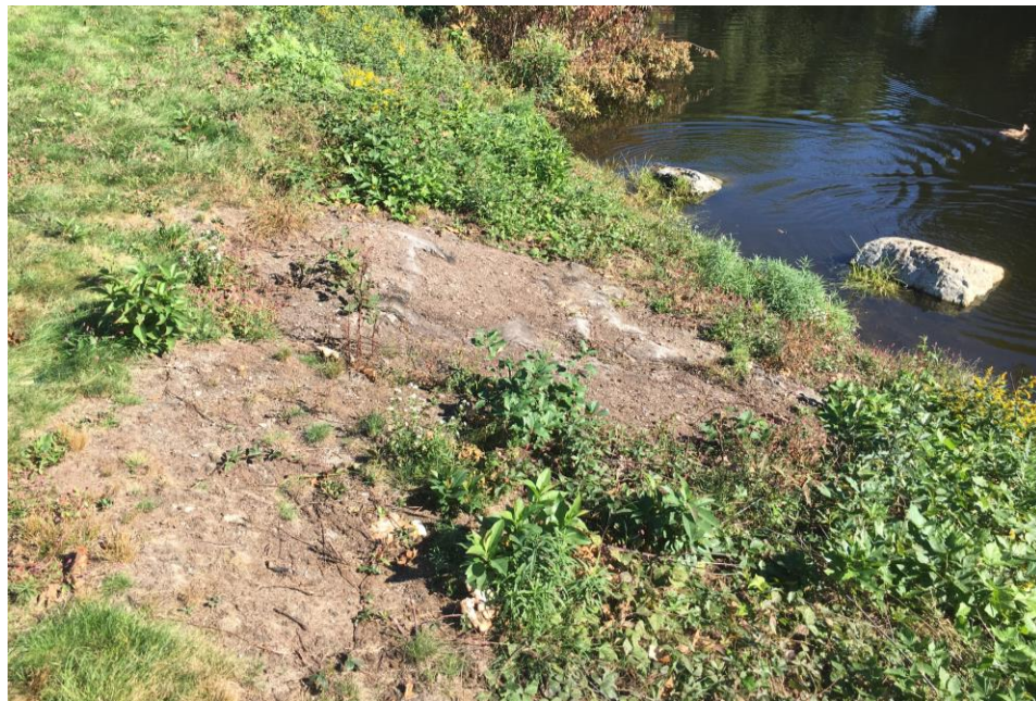
Example of eroded bank area to receive spot repair along northern pond bank..
