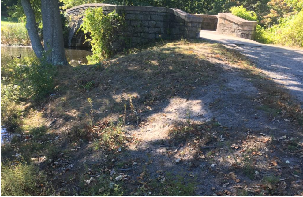
Existing compacted gravel cart path and eroded bank area.
