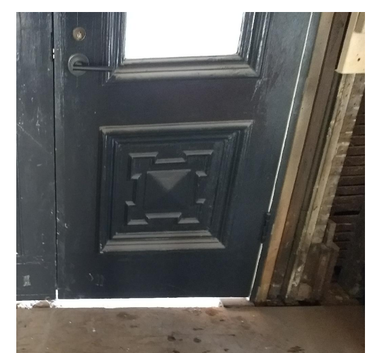
ORIGINAL CONFIGURATION HAS BEEN REVERSED: CROSSETTES CURRENTLY ON INTERIOR
