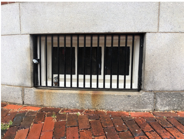
Basement window on adjacent property (162 Beacon?). Proposed black iron security grille to match this on both of our new windows.
