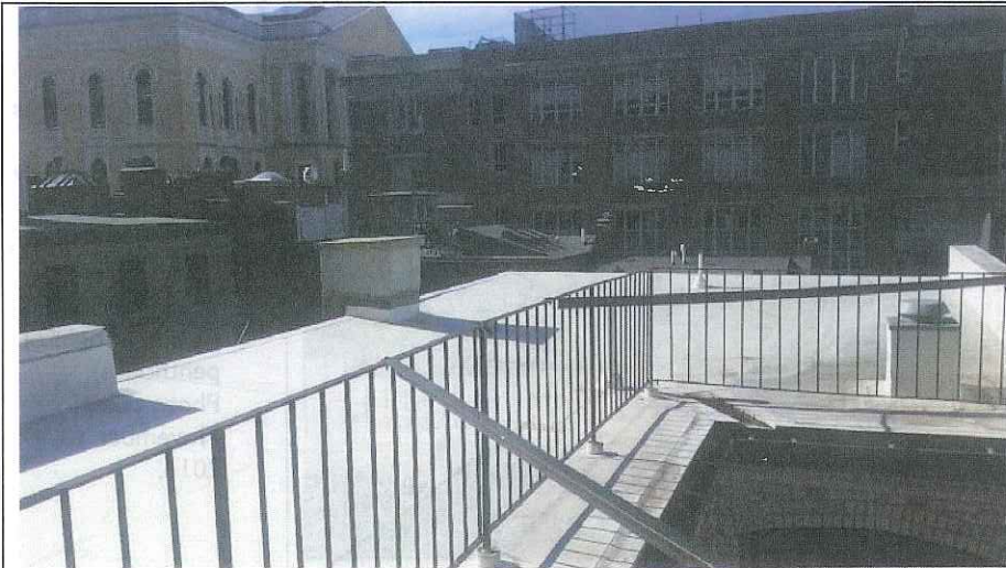
7. View west-southwest toward area of proposed steel platform (left) and southwest corner of building roof. Photo taken November 10, 2016.
