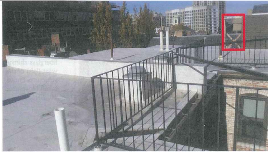
1. View northwest toward northwest corner of building roof and location of proposed Sector A antennas within proposed fiberglass chimney (red box). Photo taken November 10, 2016.
