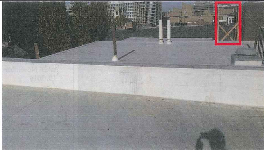
4. View north along proposed cable tray. Proposed faux chimney location indicated by red box.
