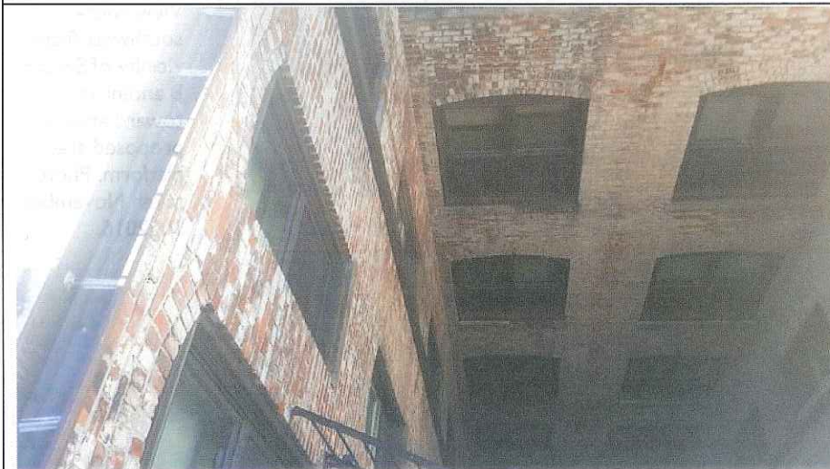
8. Location of proposed power/telco vertical run from the basement. Photo taken November 10, 2016.
