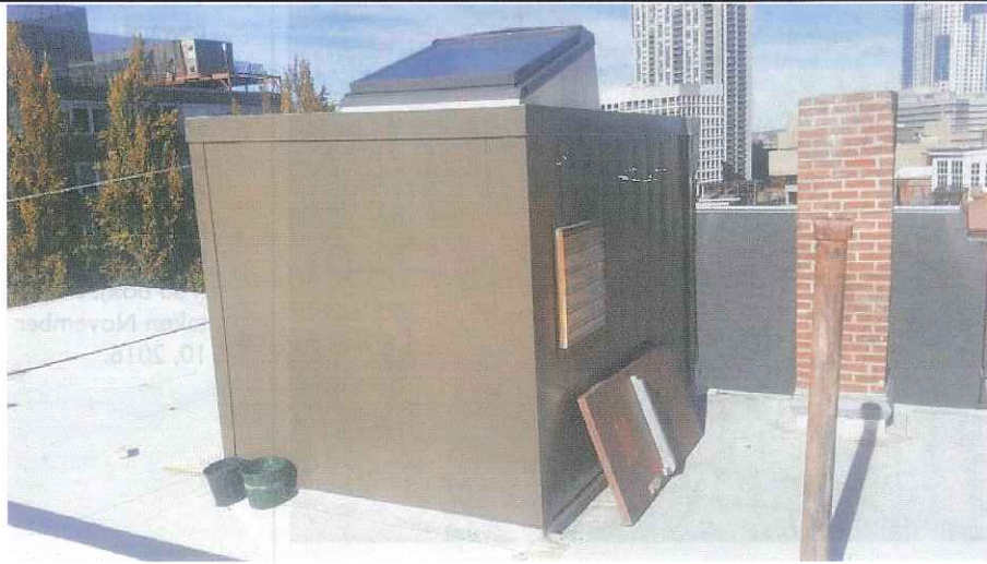
3. View north-northwest toward existing penthouse. Sector A antennas are proposed within a fiberglass chimney west (left) of this structure. Photo taken November 10, 2016.
