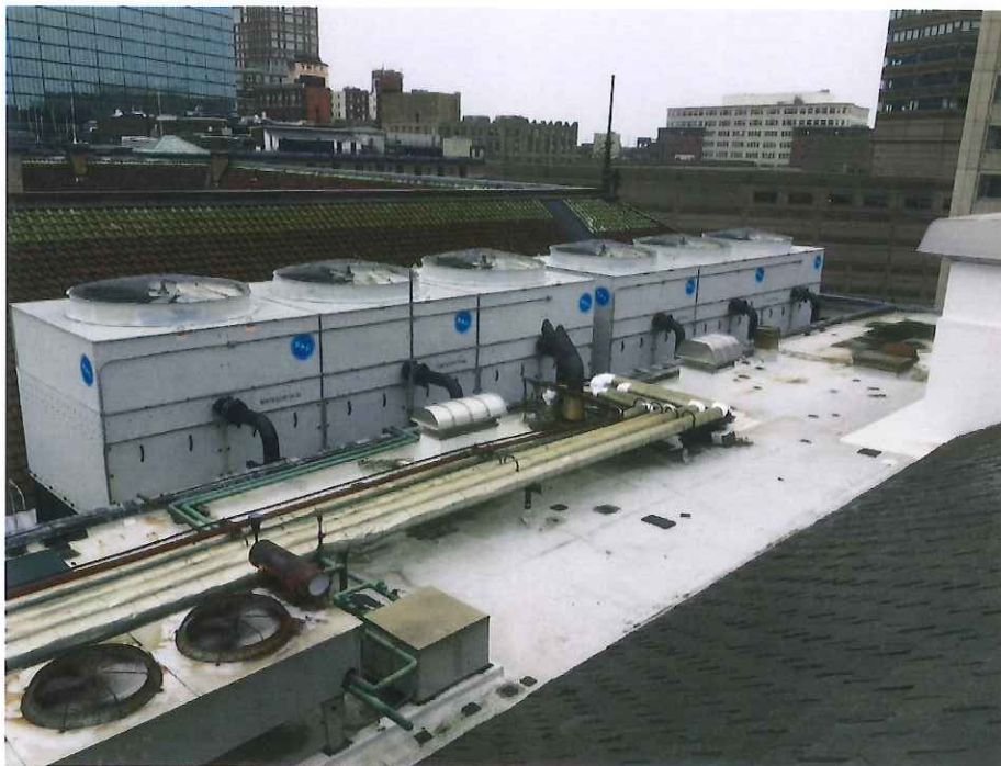
Figure 19: Johnson Building – Mechanical Equipment to remain
