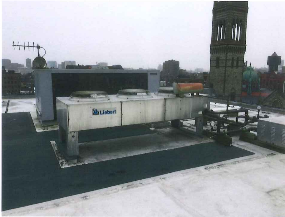
Figure 18: Johnson Building – Mechanical Equipment to be replaced by separate project.
