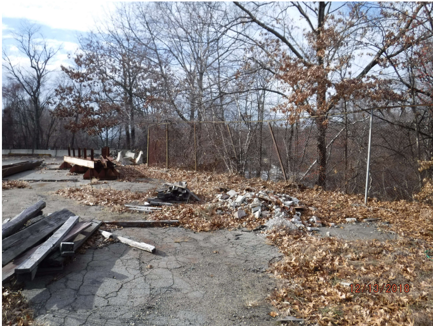
Photograph 4: Rear of the property behind the existing building near slope toward Mother Brook.
