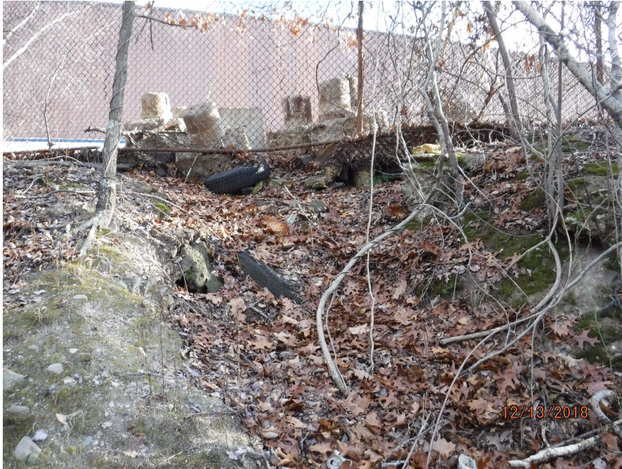
Photograph 3: Slope to Mother Brook along the rear of the property behind the existing building.
