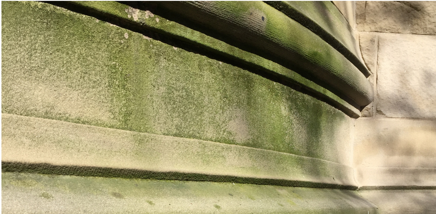
BAY NEAR FRONT ENTRY - WASH DOWN BROWNSTONE MASONRY WITH LIGHT RESTORATION CLEANER; WIRE BRUSHING, SANDBLASTING, AND OTHER ABRASIVE TECHNIQUES ARE PROHIBITED
