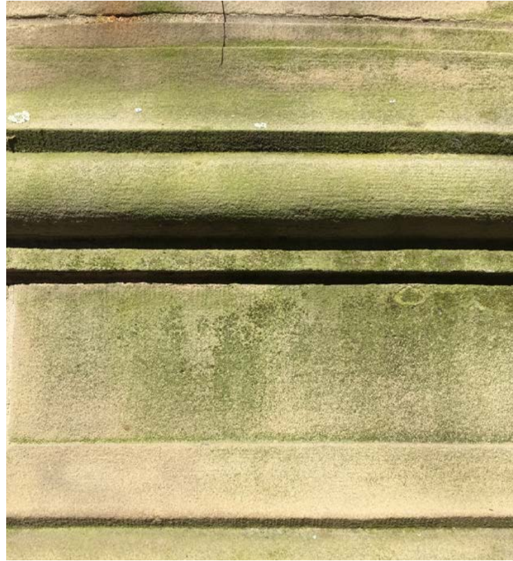
DETAIL VIEW OF FUNGAL GROWTH & MILDEW
