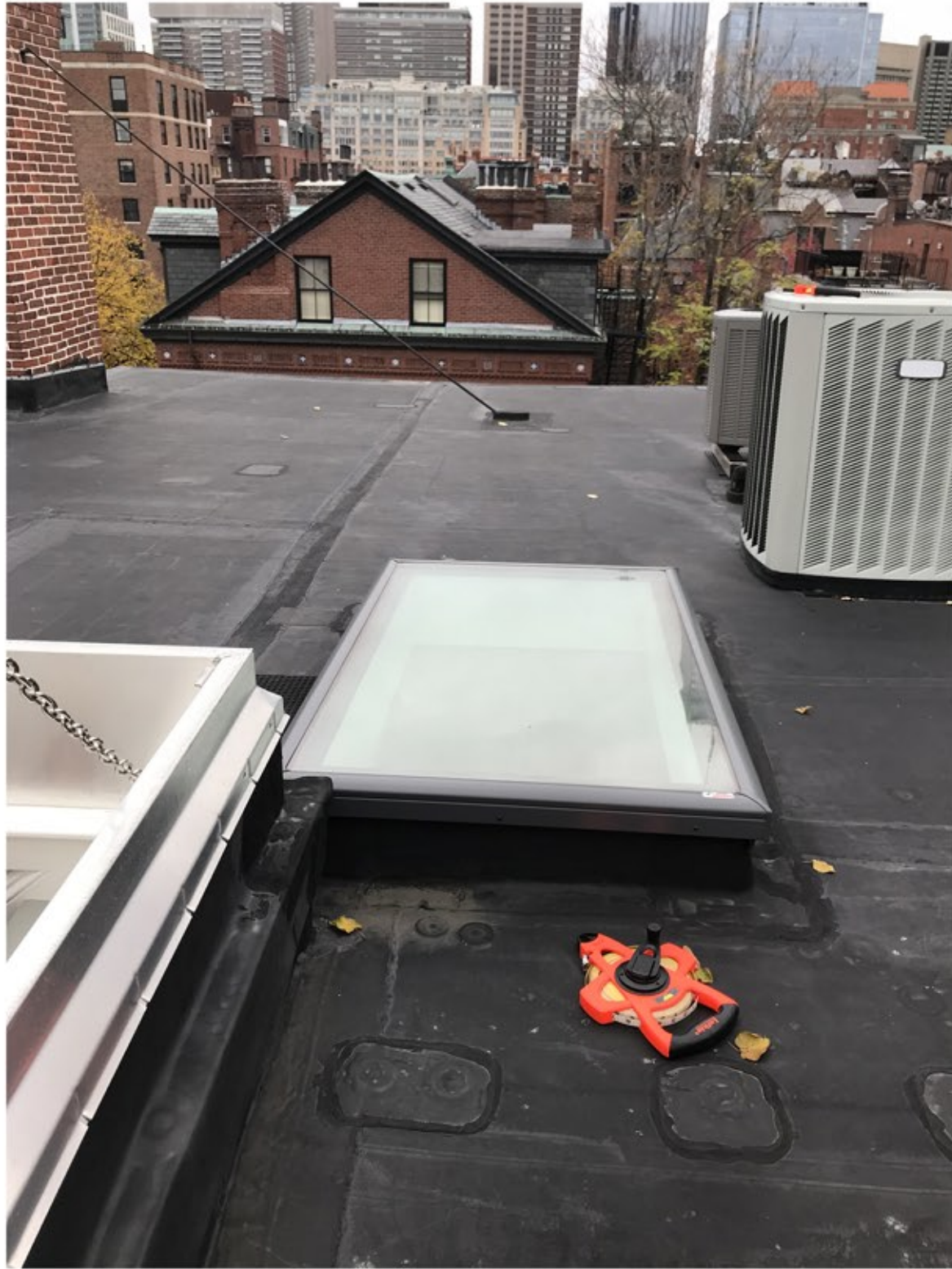
EXISTING SKYLIGHT AND A/C CONDENSERS
