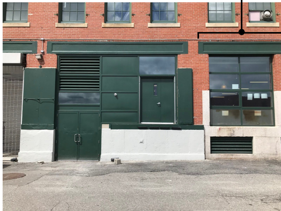
Window to be replaced
