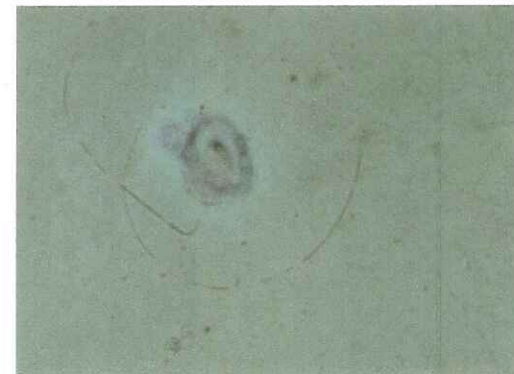
Hole in copper roof overhang needs to be repaired.
