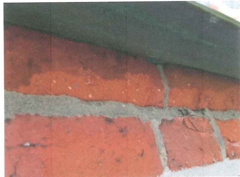
Deteriorated brick behind the parapet flashing that needs to be replaced.
