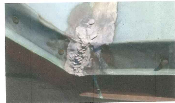
Damaged flashings with face fastening can lead to water infiltration into the roof.
