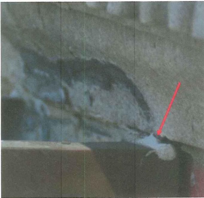
Open caulk joints at the outer face of the scuppers.
