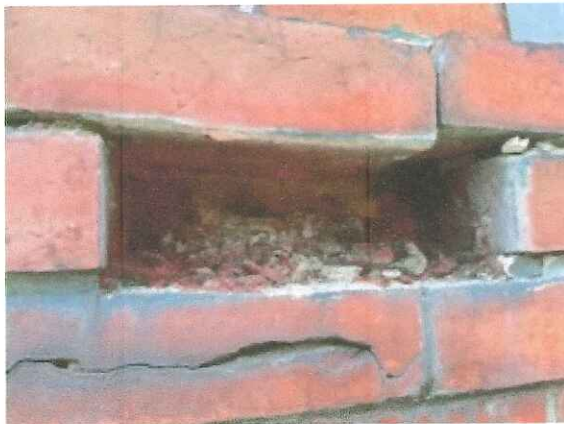
Brick had been removed by hand and the mortar has turned back to sand due to the excessive water infiltration.
