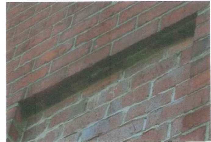
Rusted steel lintel should be removed and inset bricked in. The rust will begin to damage the wall.
