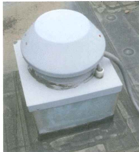
EPDM flashing should come to the top of the fan curb and have a counter flashing added.
