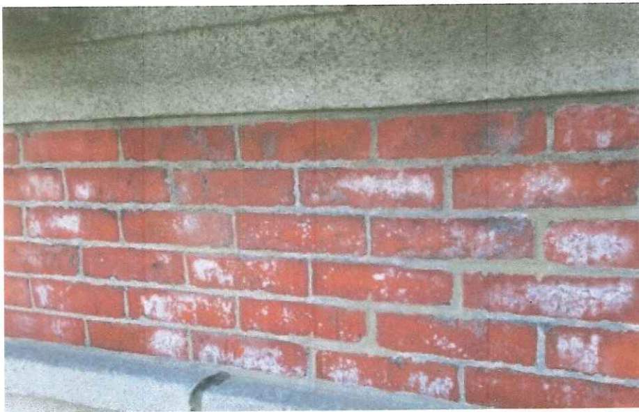
Efflorescence shows that water is getting in through the stone cornice.
