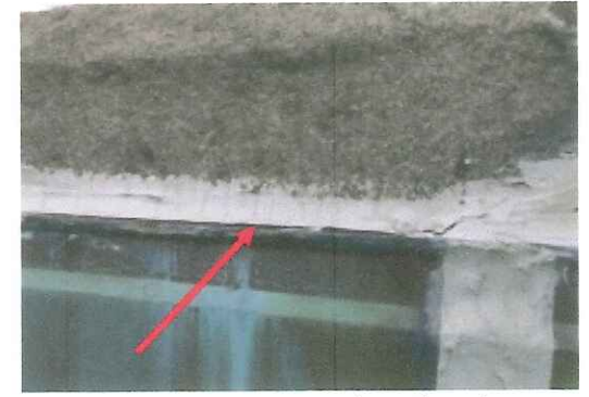
Sealant at flashing is open and needs to be re-sealed.
