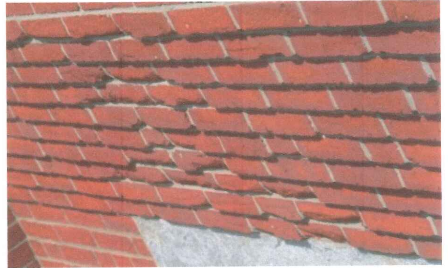
Damaged brick from fire needs to be replaced to prevent future damage.
