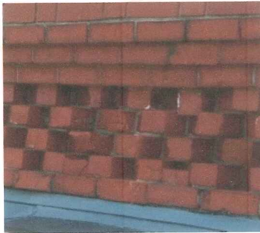
Damaged bricks at Parapet wall.
