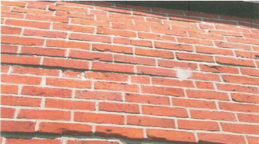
Bulge in masonry parapet needs to be rebuilt.
