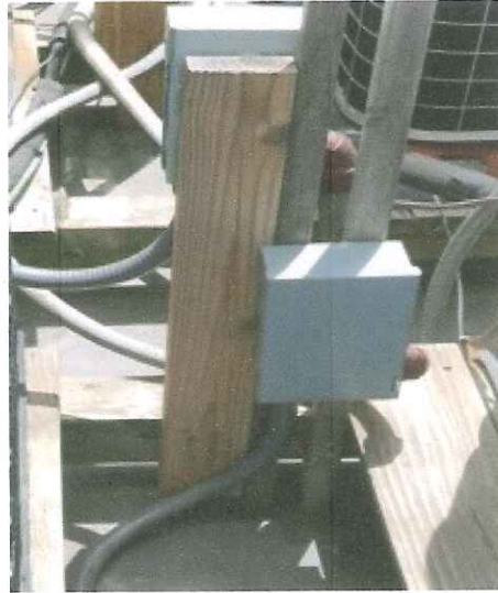
Wood is sitting directly on roof and needs to be set on sleepers and walkway pads.
