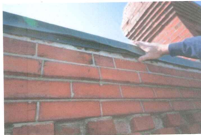
Flashing at the parapet was not installed properly an dis open to water infiltration into the wall.
