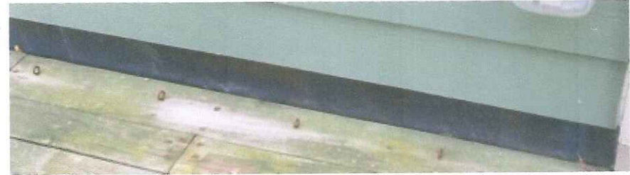
Base flashing needs to be added between siding and EPDM flashing.
