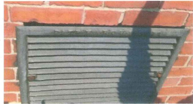
Perimeter of vent needs to be caulked.
