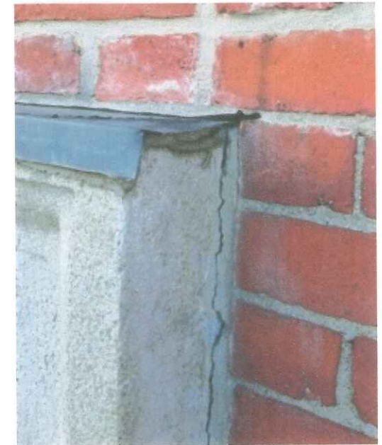
Joint between the brick and granite is cracked and should be replaced with a caulk joint.
