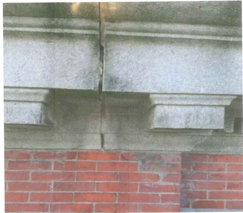
Open crack at granite cornice.
