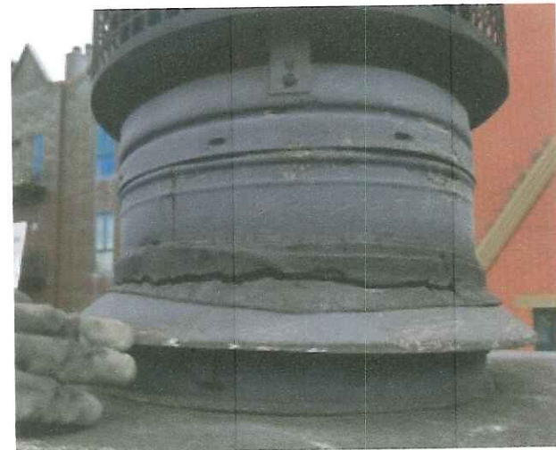
Open flange at vent needs to be re-sealed.
