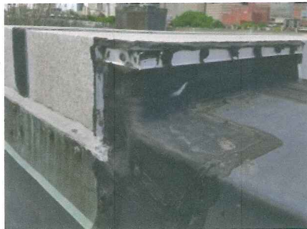
New cap flashing needs to be added.
