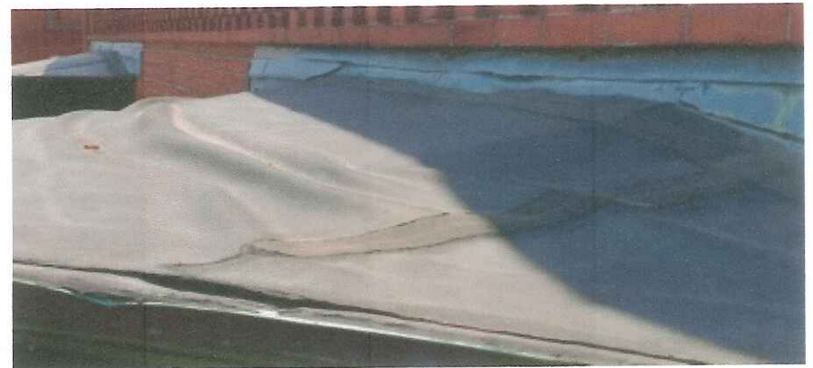
Failed EPDM roof over bay window. Roof has 2 EPDM roofs over copper.
