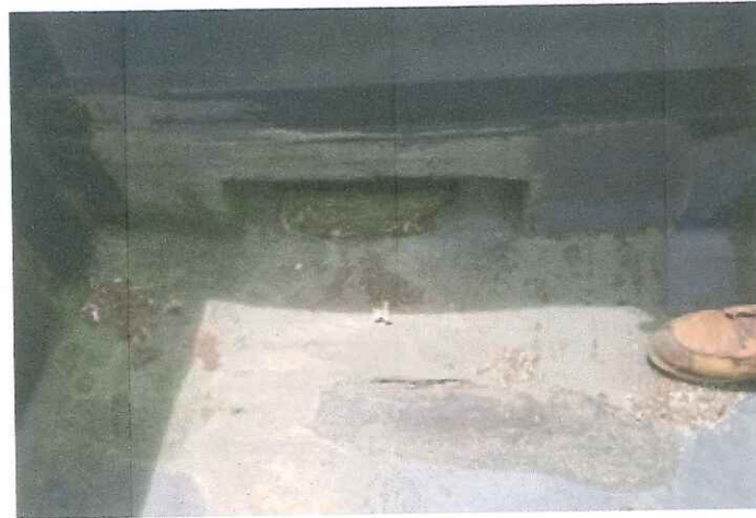
Flashing at the scupper perimeter has been patched with asphalt the is not compatible with the EPDM and will cause the EPDM to deteriorate.
