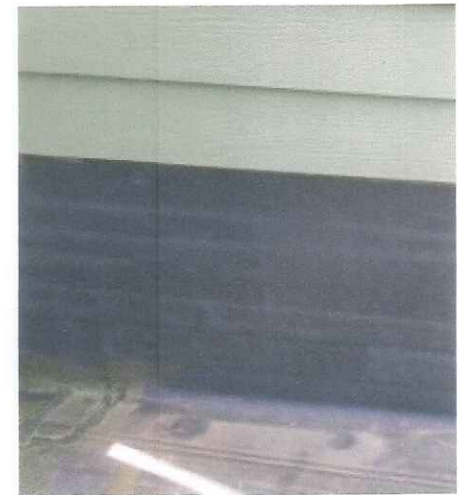
Base flashing needs to be added between siding and EPDM flashing.
