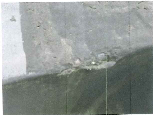
Damage at the EPDM flashing will need to be patched.
