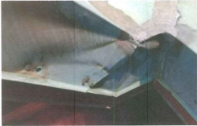
Damaged flashings with face fastening can lead to water infiltration into the roof.
