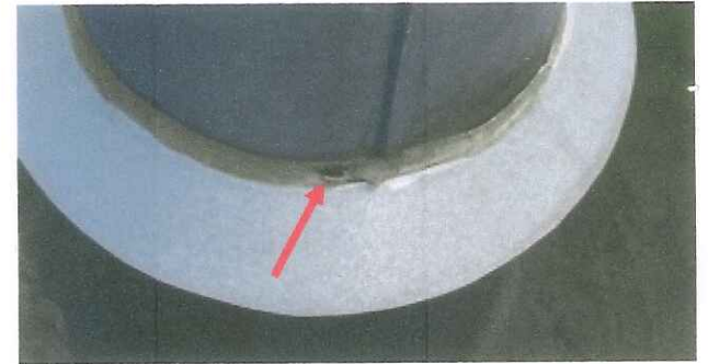
Sealant at flange is open and needs to be re-sealed.
