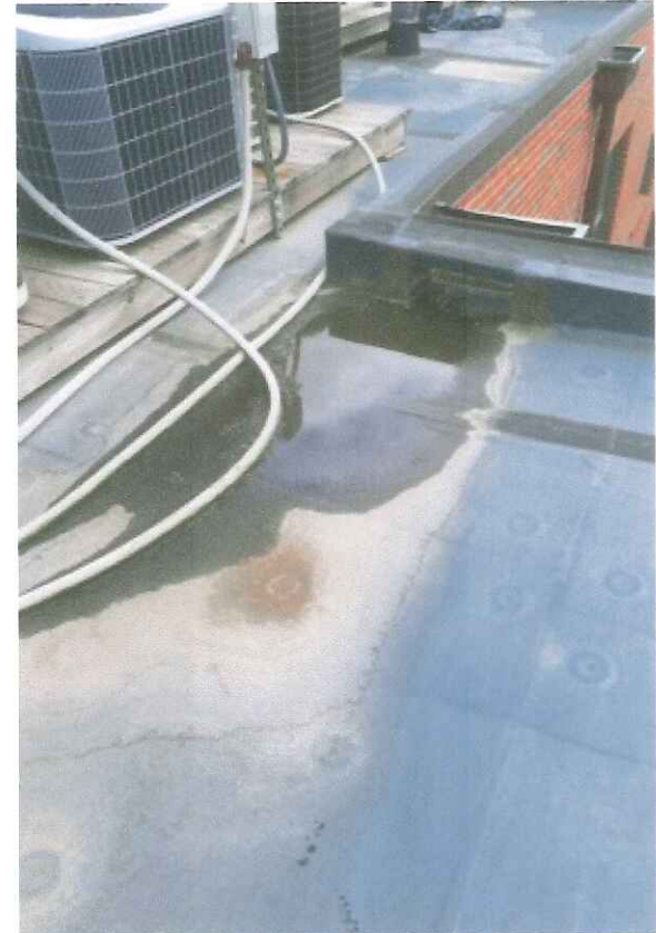
Tapered insulation should be added to create more of a taper for proper drainage.
