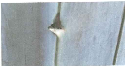
Damage at copper at vent stack needs to be repaired.
