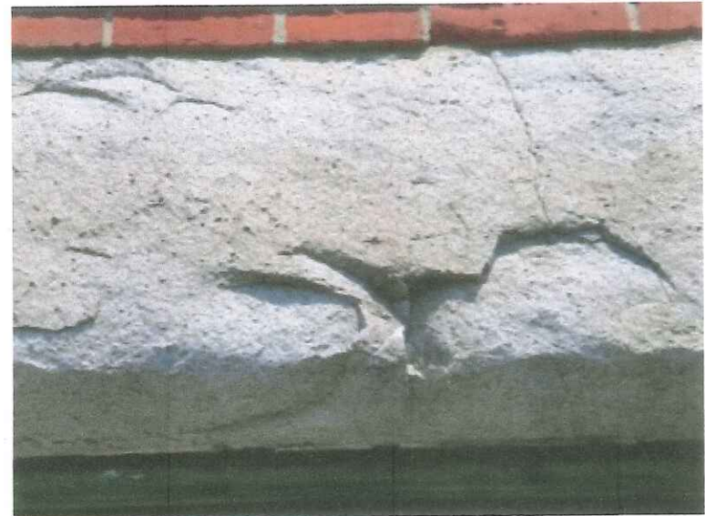
Damaged granite window header needs to be replaced.
