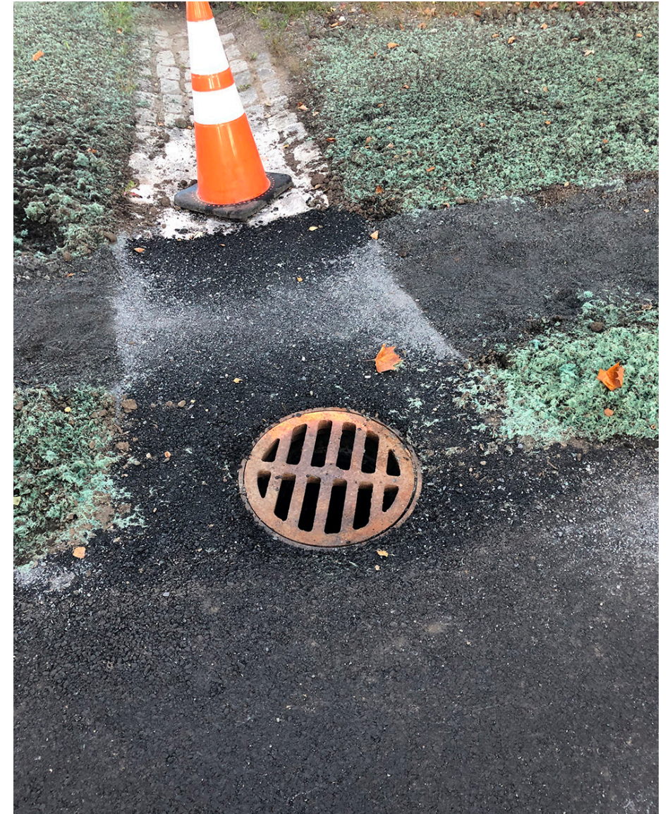
Example of a new cobblestone spillway nearing completion. Proposed spillway would be constructed in the same way.
