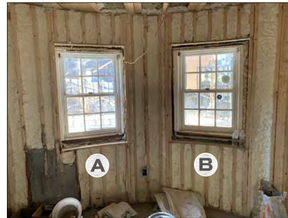
9 Exhibit - Existing non-original windows; interior view at Garden Floor
