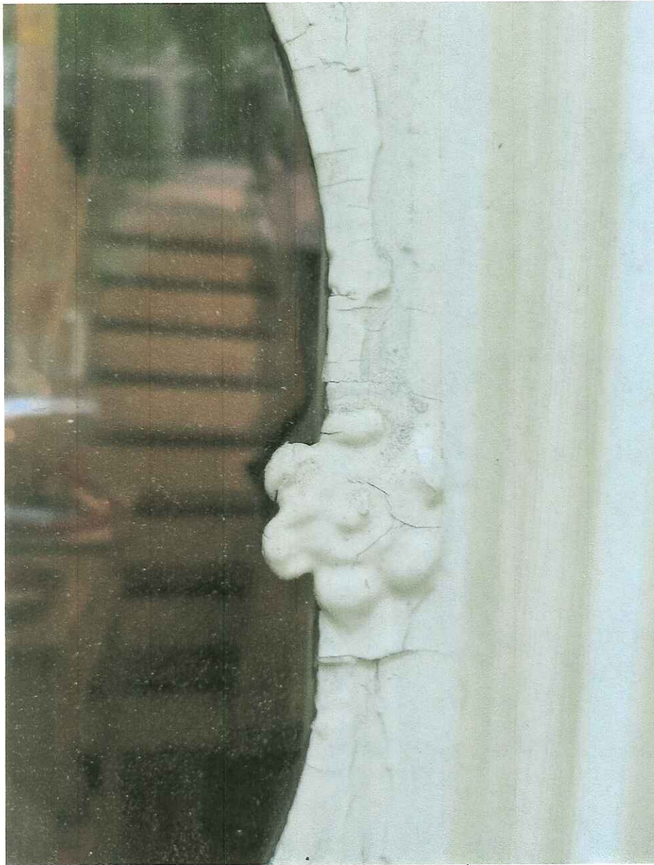
gunked lead window detail 8th Mt. Vernon St.
