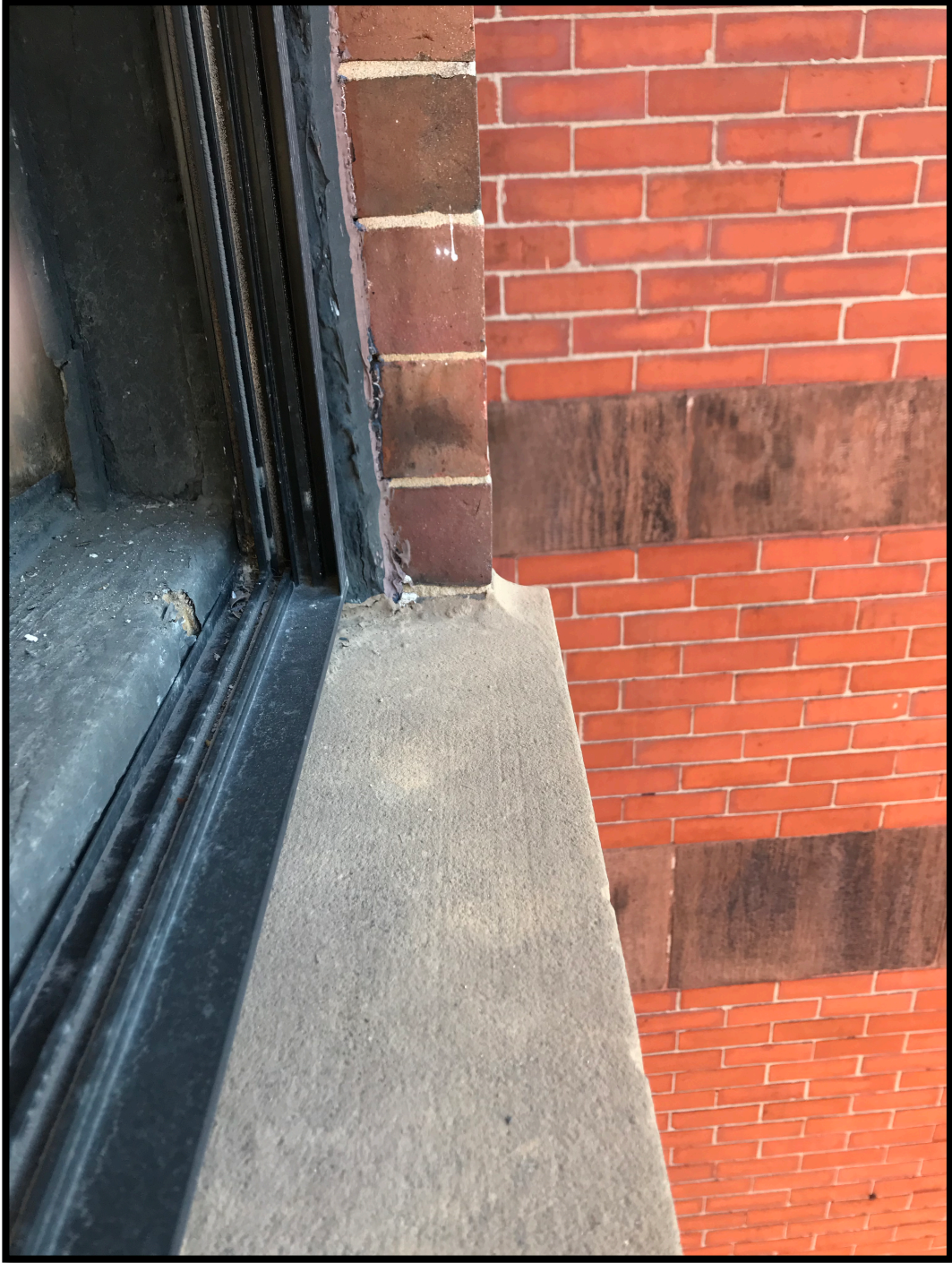
Existing Triple-Track storms on too-short sill
