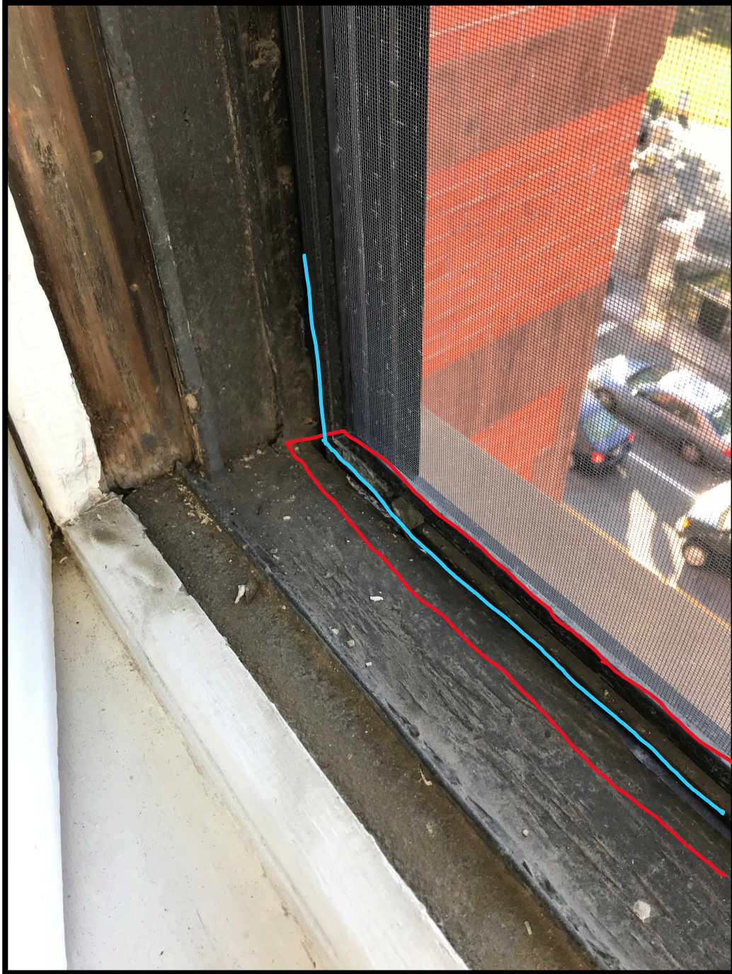
Proposed sill extension (Red) into existing Brick Mold Proposed location of storm window bottom edge (Blue)
