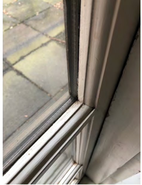
Clear Insulated Glass from 1997 at Rear Facade; Dark Aluminum Spacers Used Due to Brown Exterior
