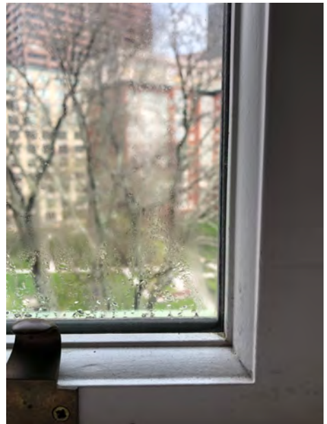
Detail of Water Droplets and Trapped Moisture on Inside of Insulated Glass Where Seals Have Failed
