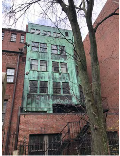
First Floor Brick with 6/6 True-Divided Light Sash; Copper Cladding at Floors 2 Thru 9 with 1/1 Windows
