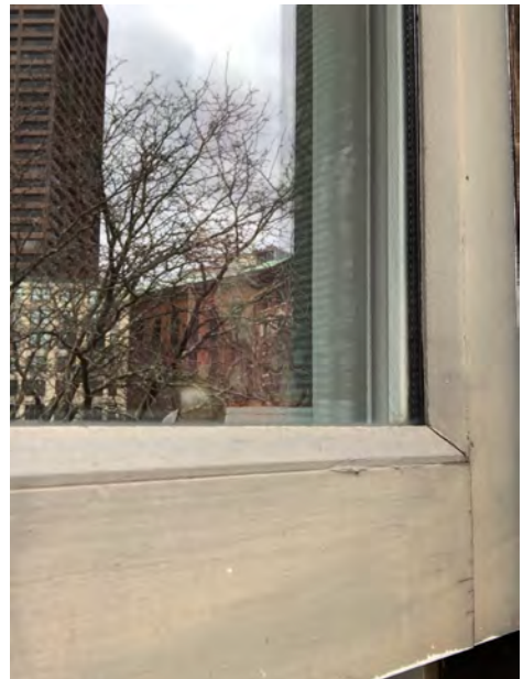
Exterior Detail of Wood Putty Glazing Profile at Double-Hung Window of Rear Facade
