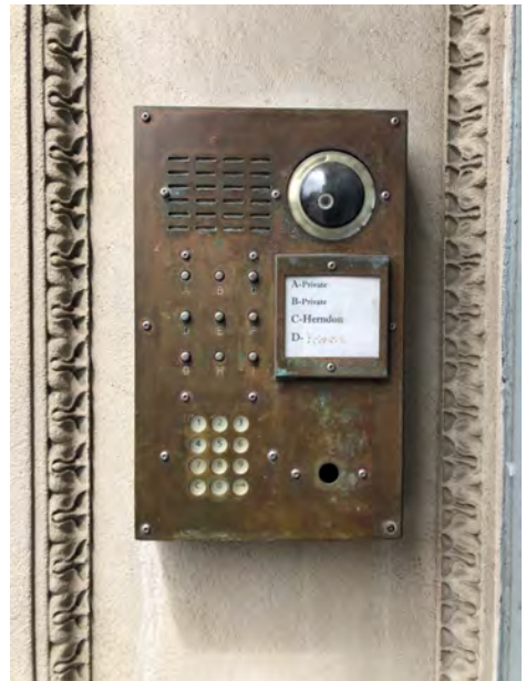
Existing Circa Video Door Intercom System Installed in 1997 on 1918 Limestone Surround
