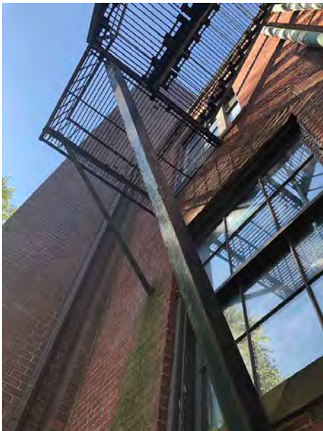
Large Angled Bracket to be Removed; Replacement Support to be Vertical
