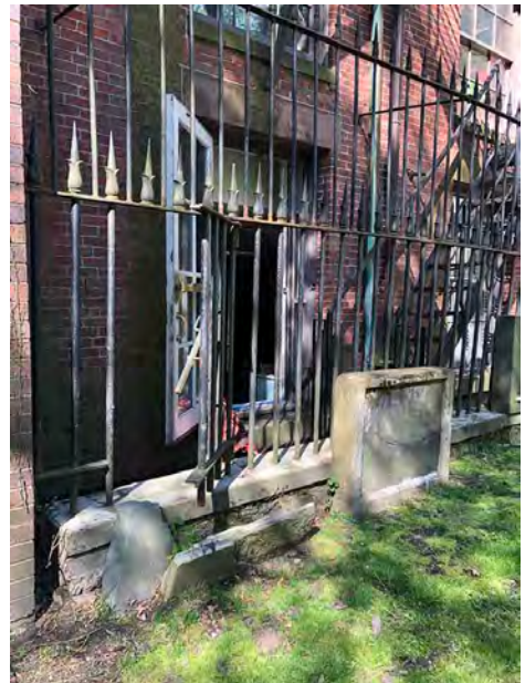
Swing Gate Incorporated Into Fence at Fire Escape Exit
