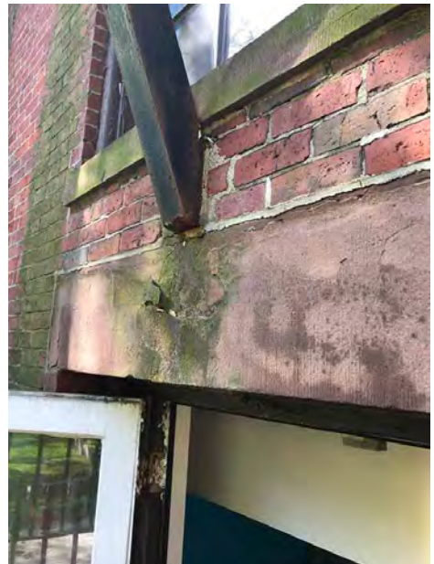
Base of Bracket Embedded in Narrow Masonry Band; Removal Will Protect Brownstone and Brickwork
