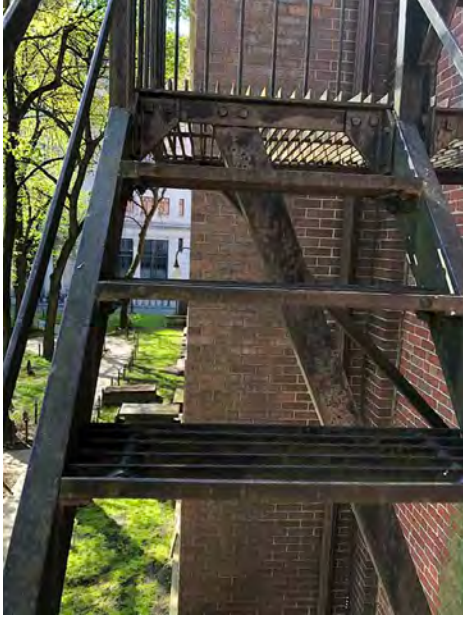
Upper Portion of Angled Bracket at Third Floor Landing; Smaller Bracket Beyond to Remain in Place; Larger Bracket in Foreground to be Replaced
