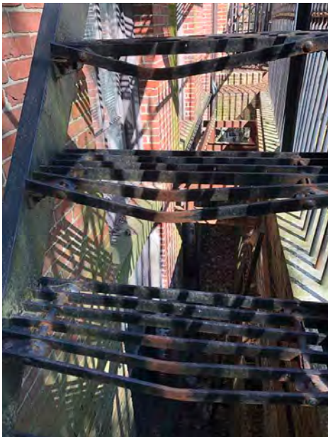
Bent Stair Tread Gratings to be Repaired
