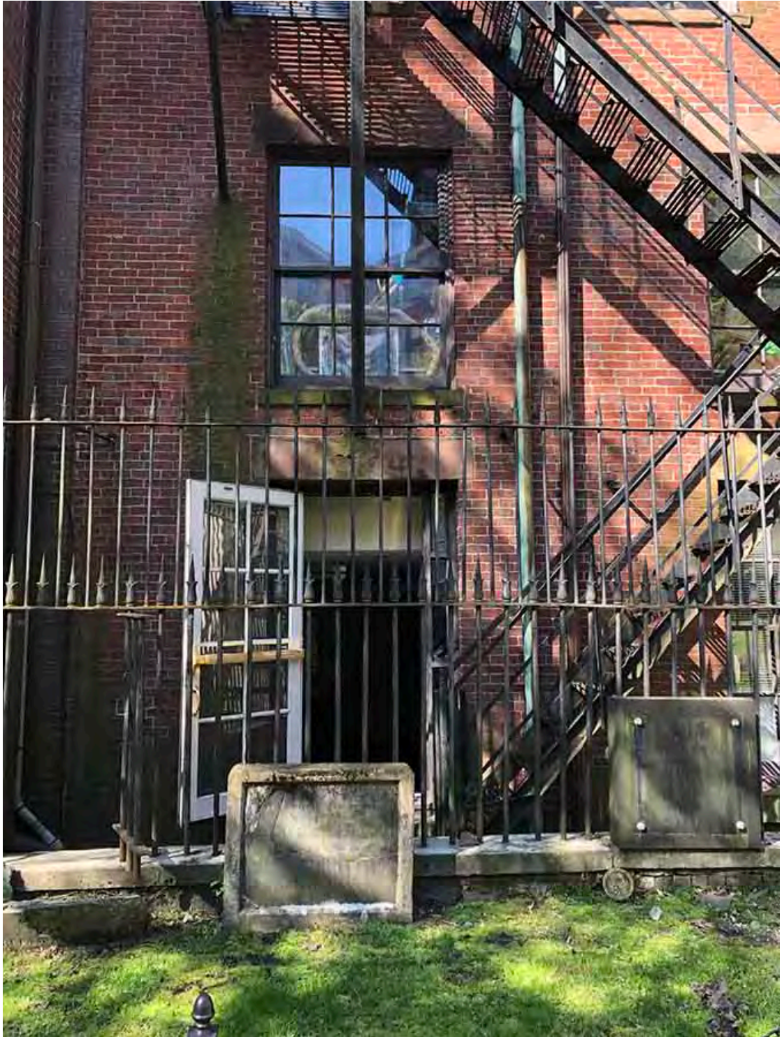
REAR FACADE AT EXIT LEVEL OF FIRE ESCAPE TO GRANARY BURYING GROUND; REPAIRS TO BE PROVIDED BEHIND EXISTING FENCE AT AREAWAY
