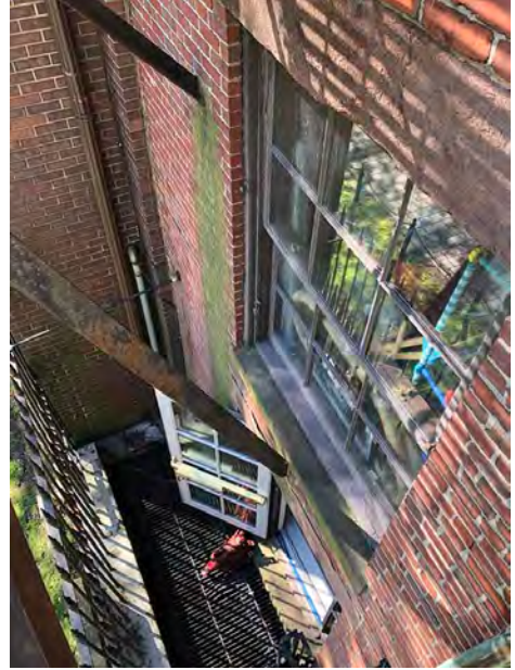
Angled Brackets Supporting Third Floor Landing; Smaller Bracket to Remain; Larger Bracket to be Replaced with Vertical Support to Match
