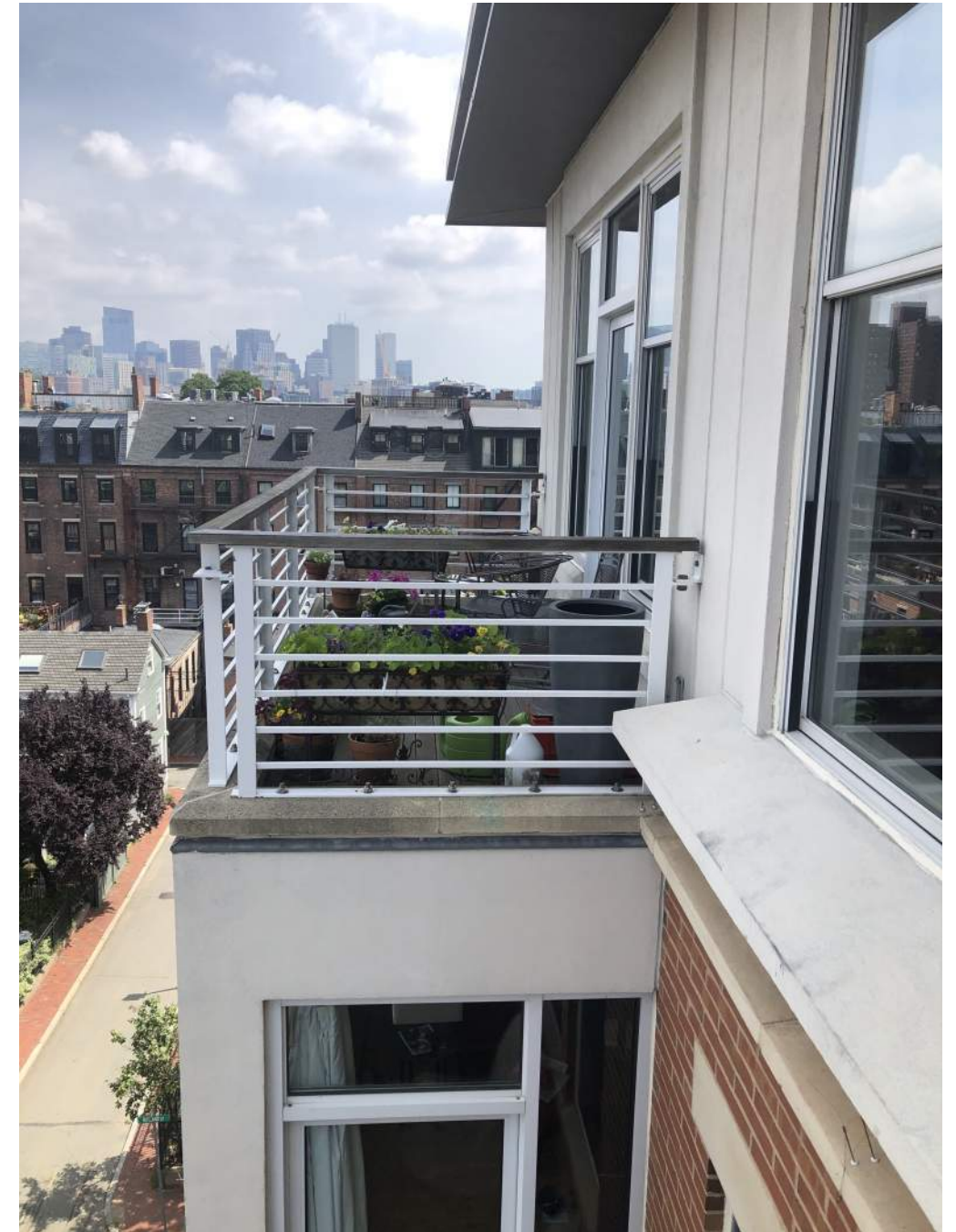
TYPICAL EXISTING WINDOWS and TERRACE DOOR 6th Floor Terrace - Rear Alley View
