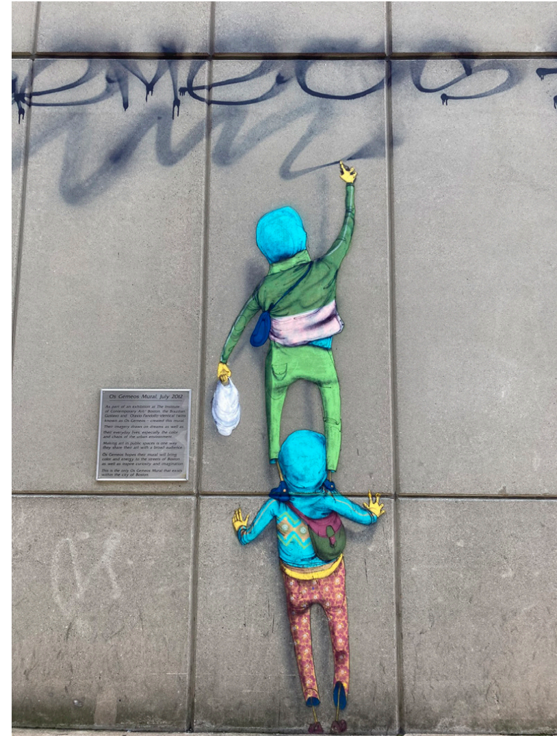
Detail View of Existing Graffiti on Garage Egress (To be preserved and lit)
