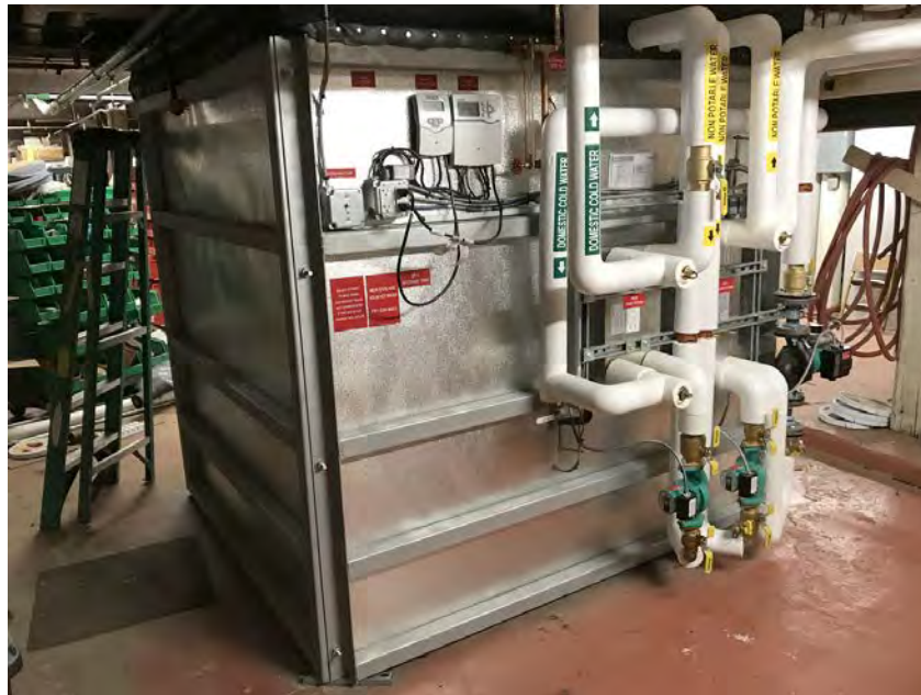
Typical EverStor Tank w/ controls
