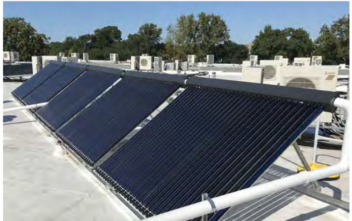
Example similar installation (5'-6" height overall.)
