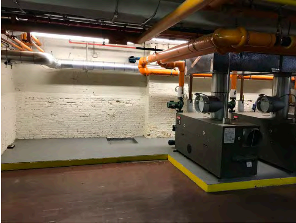
Area for Solar Tank in Basement Mech. Room
