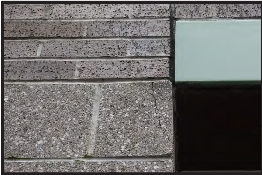
STEEL LINTEL AT WINDOW IS RUST JACKING THE MASONRY, OPENING THE BUILDING FACADE FOR WATER AND FREEZE THAW DAMAGE.
