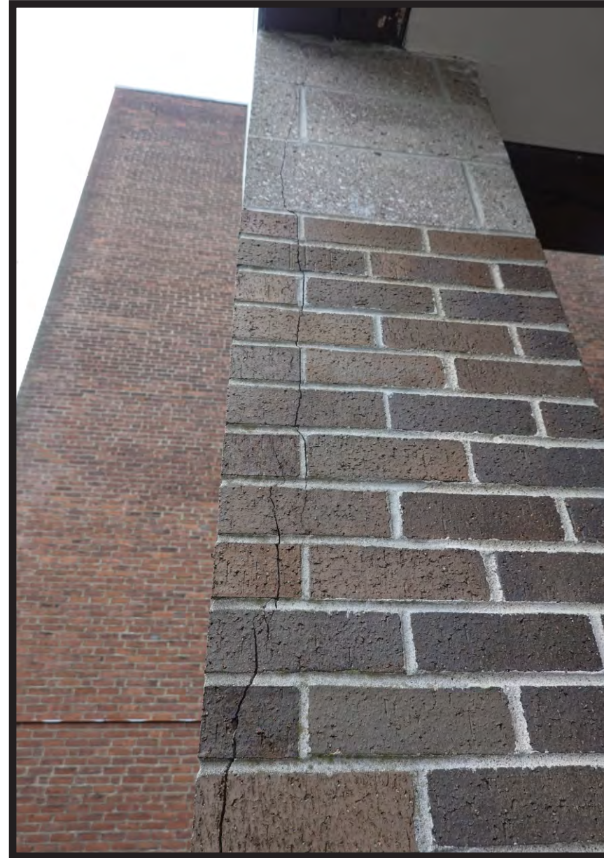
FREEZE THAW FROM ABOVE DAMAGE / RUSTING OF STEEL MEMBERS. OPENING THE BUILDING FACADE FOR WATER AND FREEZE THAW DAMAGE.
