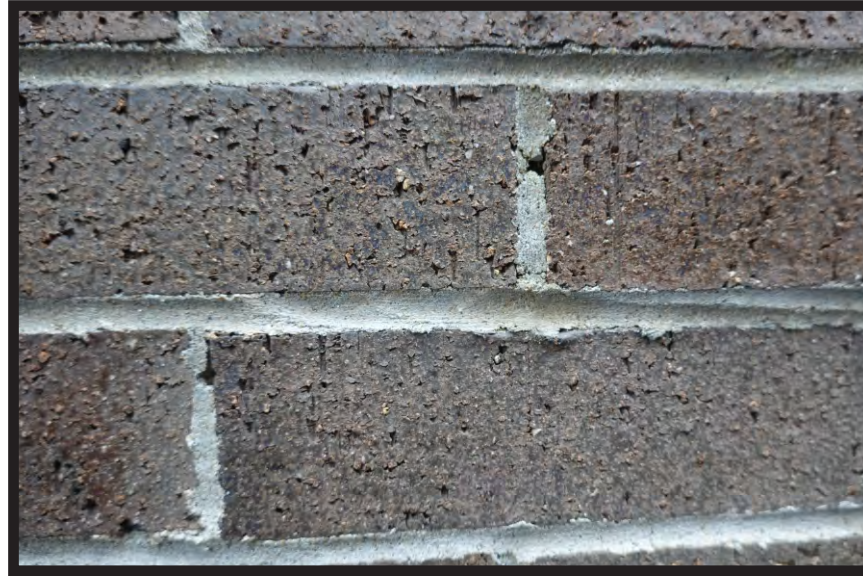
FAILED MORTAR JOINTS, OPENING THE BUILDING FACADE FOR WATER AND FREEZE THAW DAMAGE.
