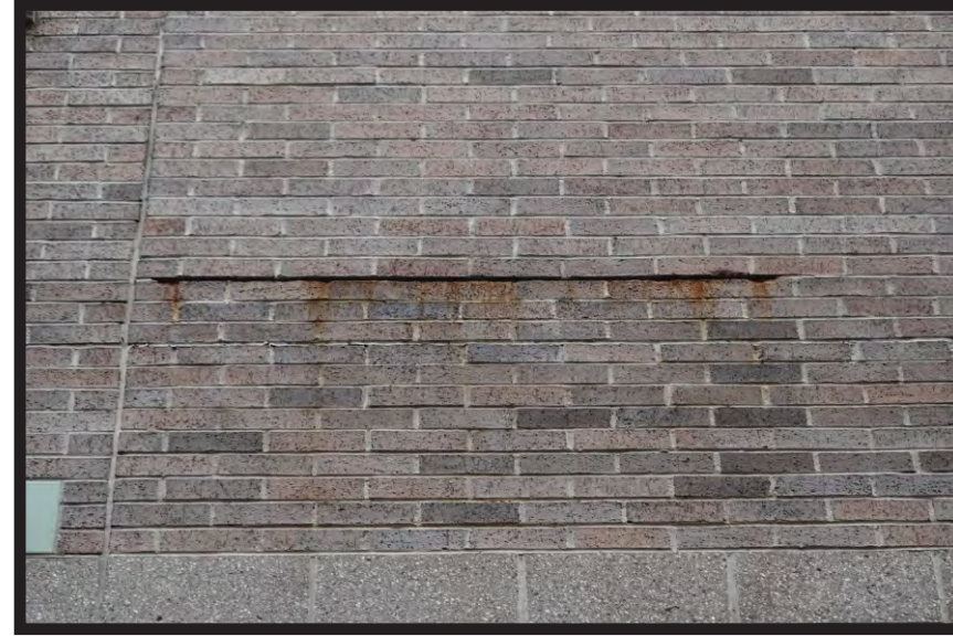
STEEL LINTEL IS RUST JACKING THE MASONRY, OPENING THE BUILDING FACADE FOR WATER AND FREEZE THAW DAMAGE.
