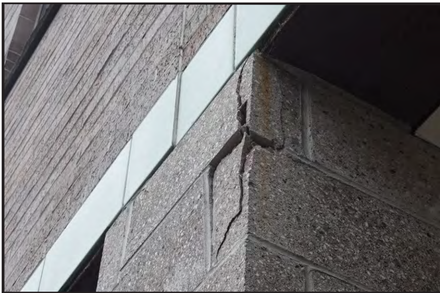
STEEL LINTEL IS RUST JACKING THE MASONRY, OPENING THE BUILDING FACADE FOR WATER AND FREEZE THAW DAMAGE.
