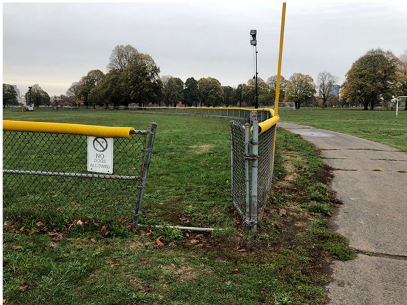
MISSING/DAMAGED FENCES, SCOREBOARDS, ETC
