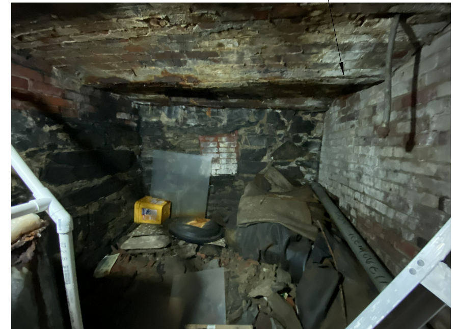
PHOTO OF END WALL OF VAULT UNDER ENTRY STAIR/WALK, LOOKING TOWARD BERKELEY ST.
