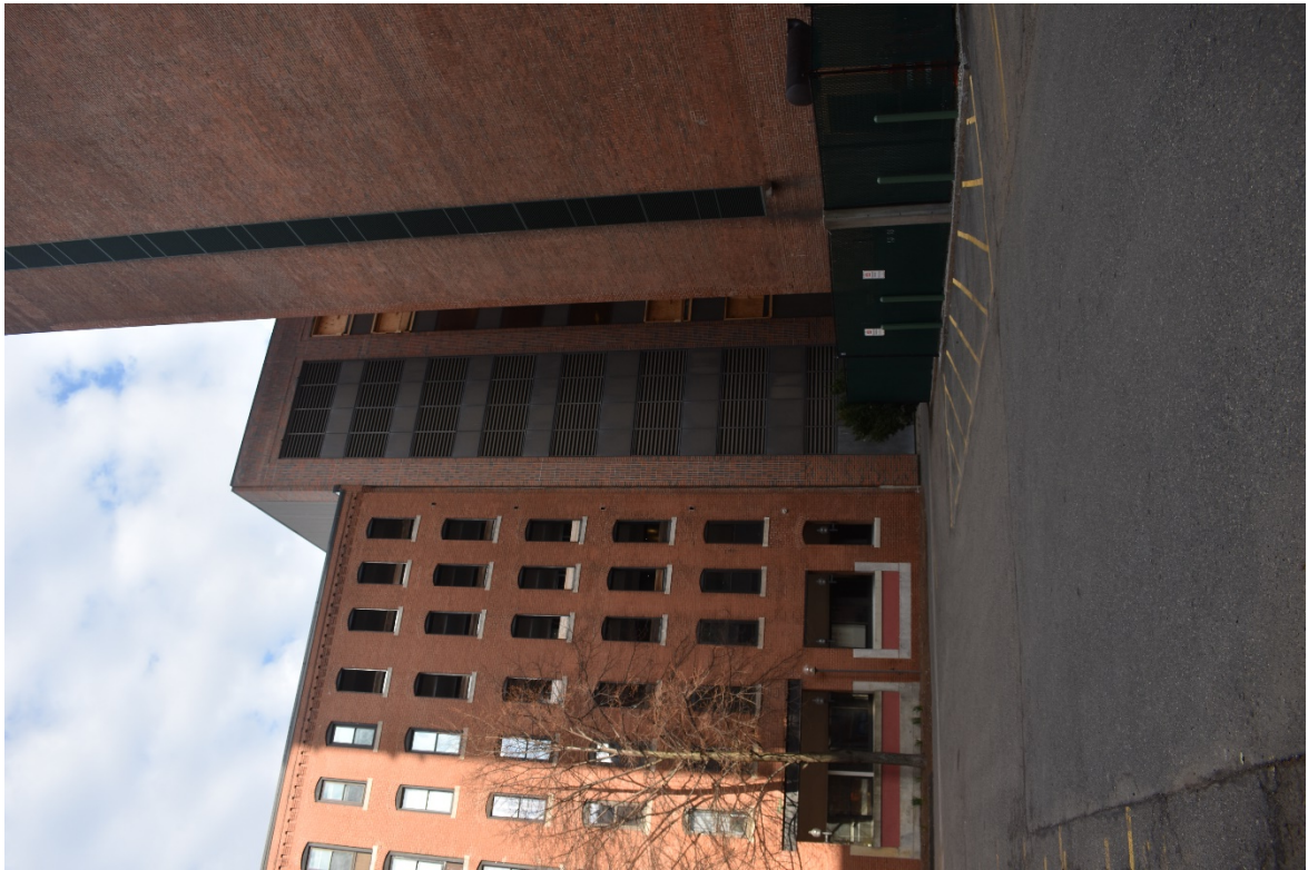
11. Rear (east) elevation of building from Farnsworth Street. 51 Sleeper Street is at the center of the photograph; one of the lower metal panels and louvers proposed for replacement with metal maintenance door for access to rooftop equipment.
