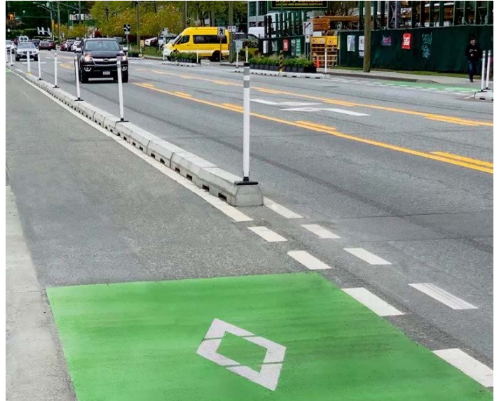
Example of concrete curbing and flexposts used to separate a bicycle facility from a vehicular travel lane. The spacing of the curbing pieces and flexposts will vary along the length of Massachusetts Avenue.
