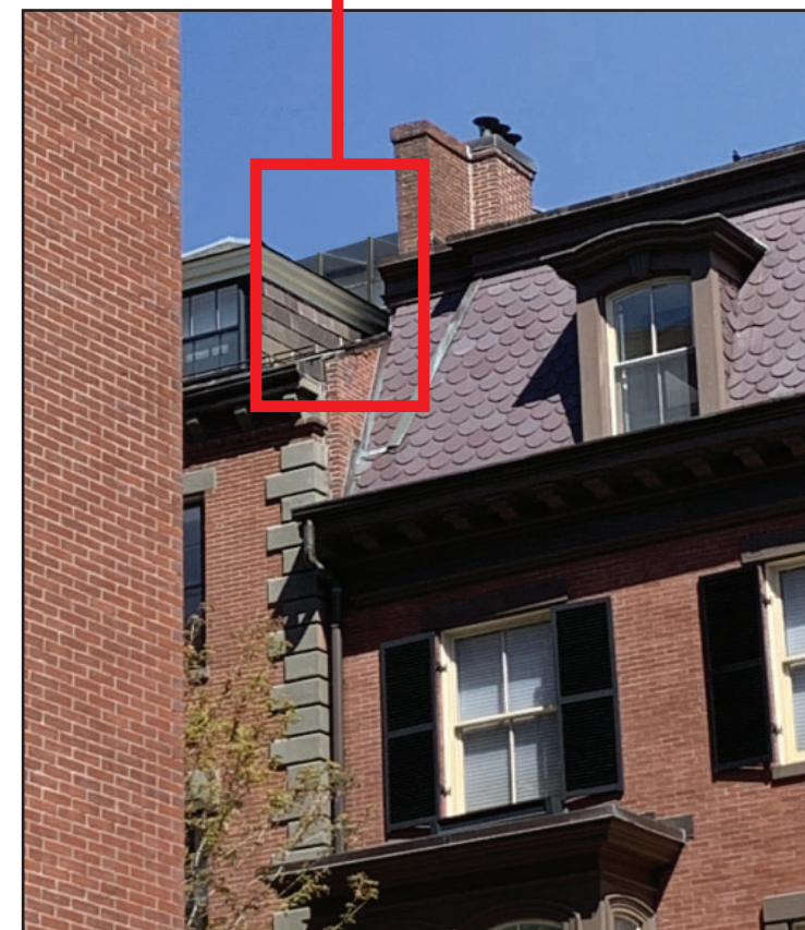
A View from Pinckney Street looking up at an altered photo showing the new bronze square frame of the glazed head house skylight.
