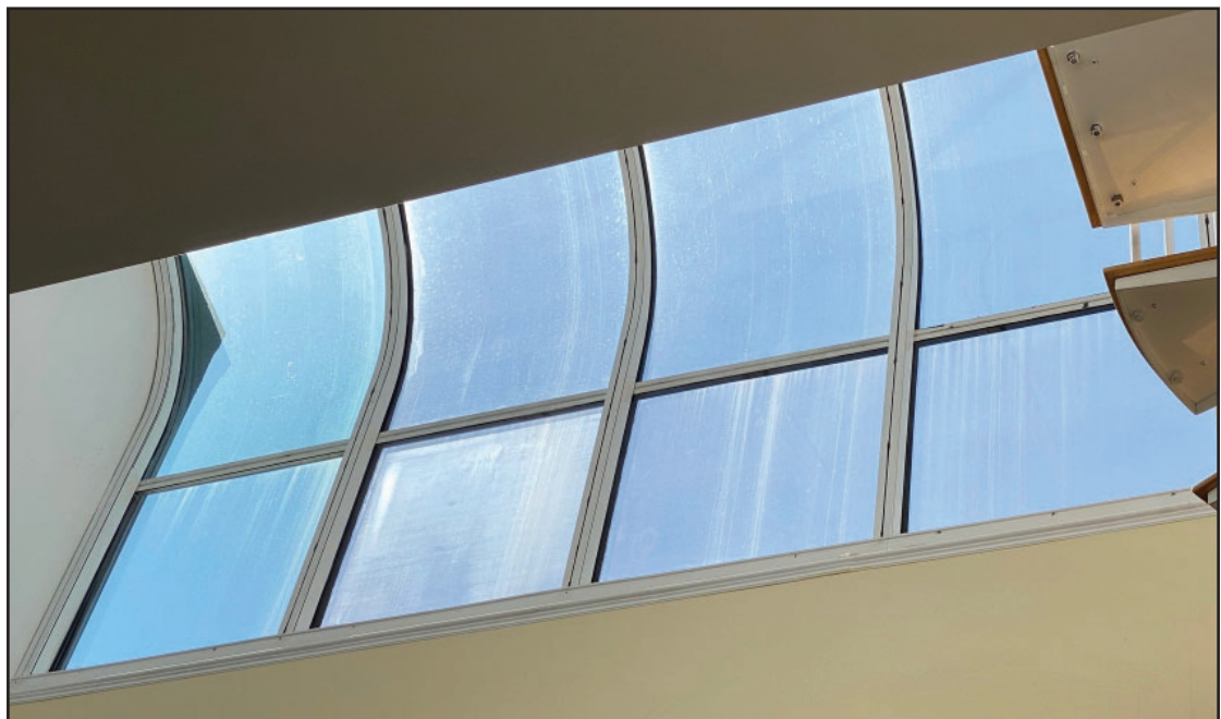
Broken seals with condensation in panes. Photo taken from inside, looking up.
