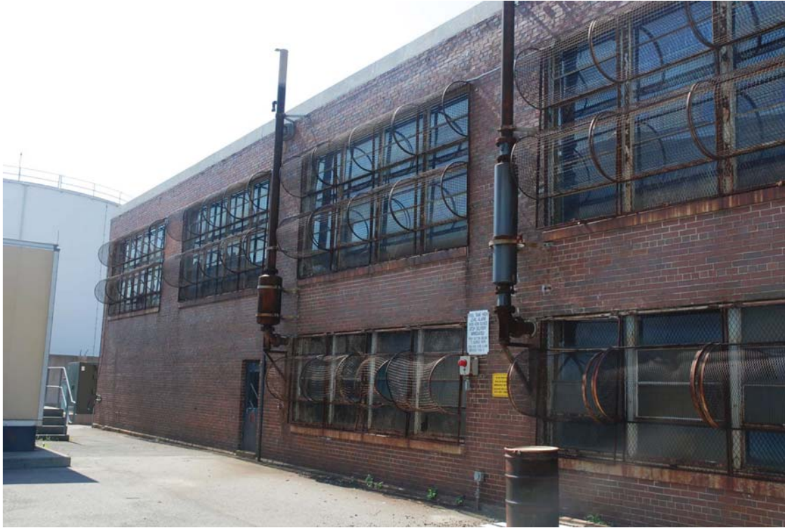
7. Former Logan Airport Pumping Station, 161 Prescott Street, Boston, MA. View of rear (E) elevation, detail of windows, photographer facing SE, August 2019.
