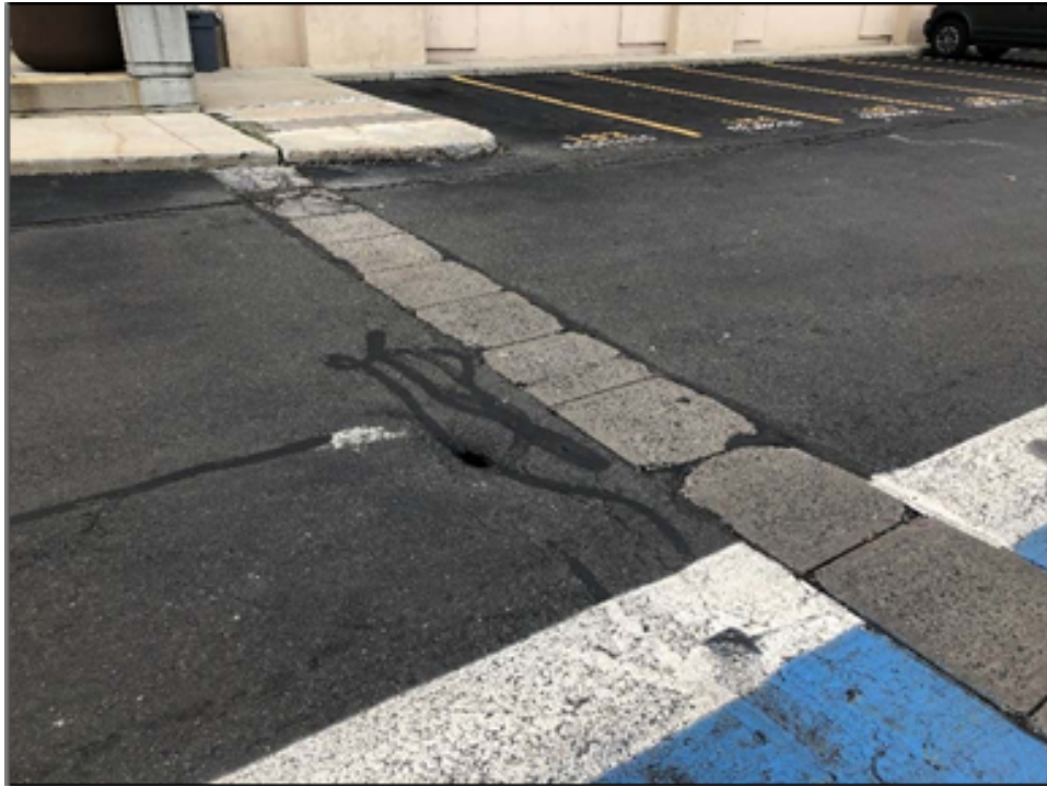
Above: Sinkhole Location
