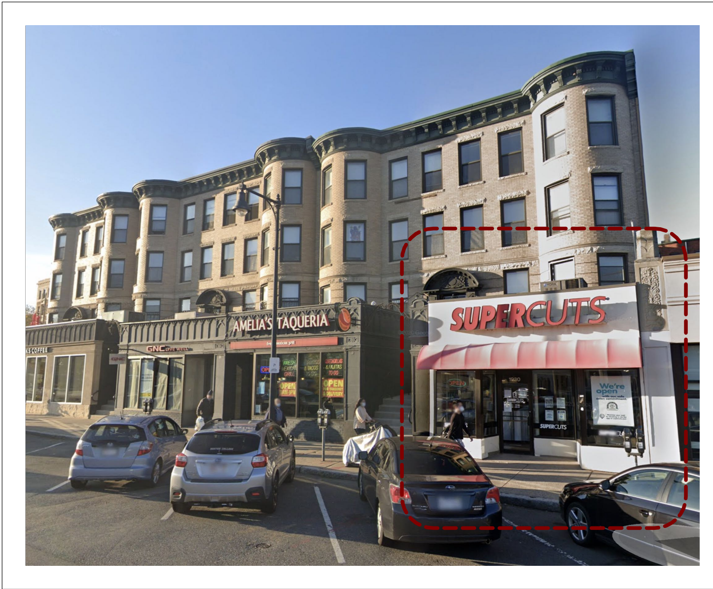
LOOKING N/W ALONG BEACON STREET STOREFRONT RENOVATIONS TO MATCH: GNC & AMELIA'S TAQUERIA STOREFRONT
