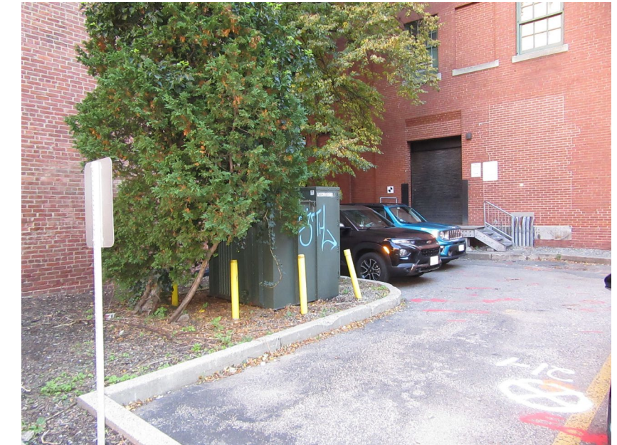
6. 11 Sleeper Street transformer, view northeast
