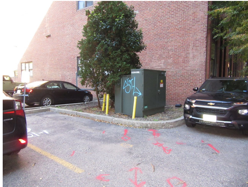
5. 11 Sleeper Street transformer, view northwest
