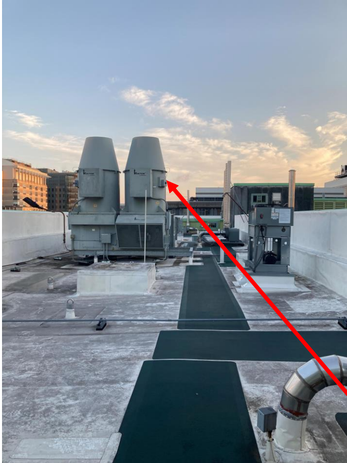
Example of existing equipment (to remain)
