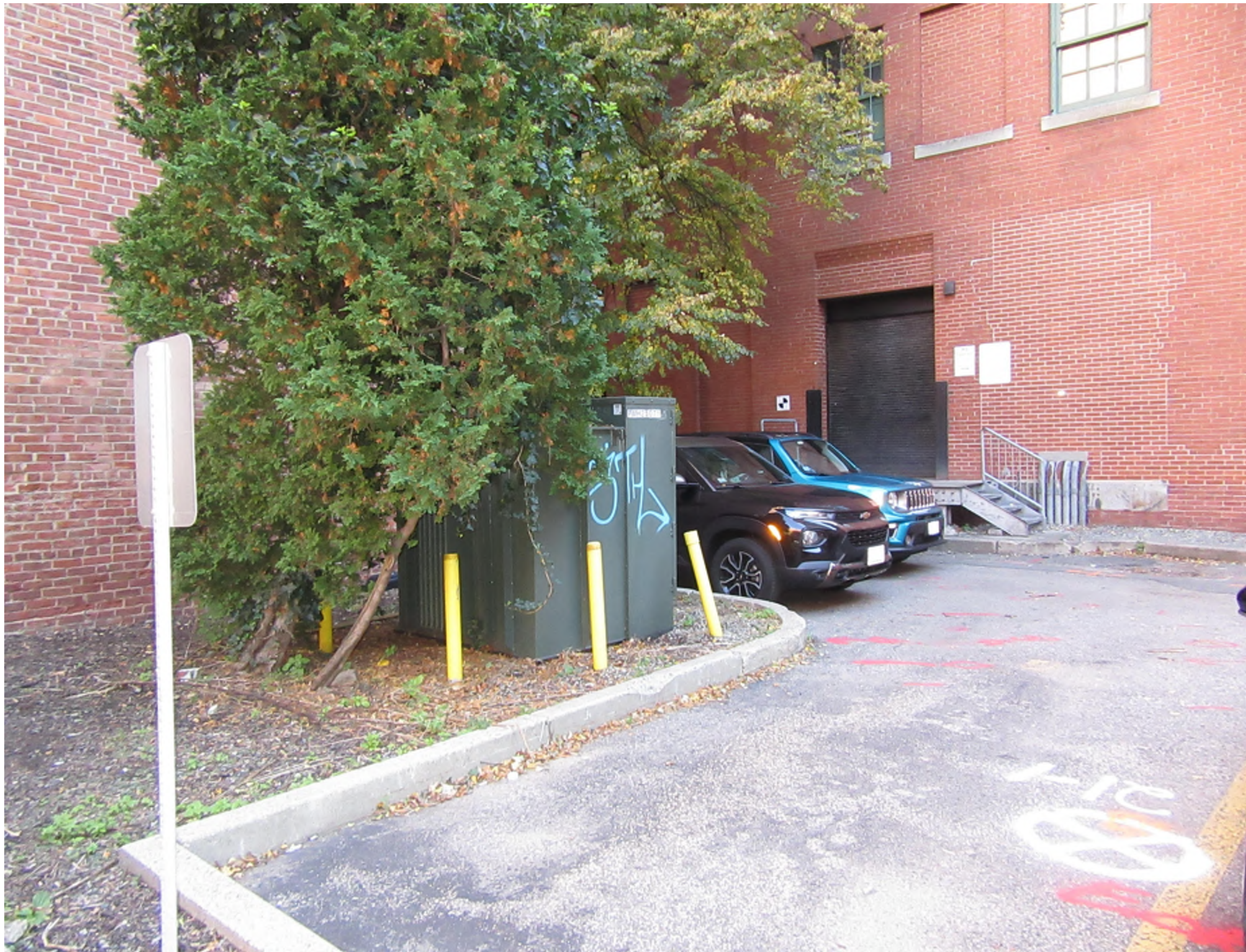
PHOTO 6 - 11 SLEEPER STREET TRANSFORMER - VIEW NORTHEAST
