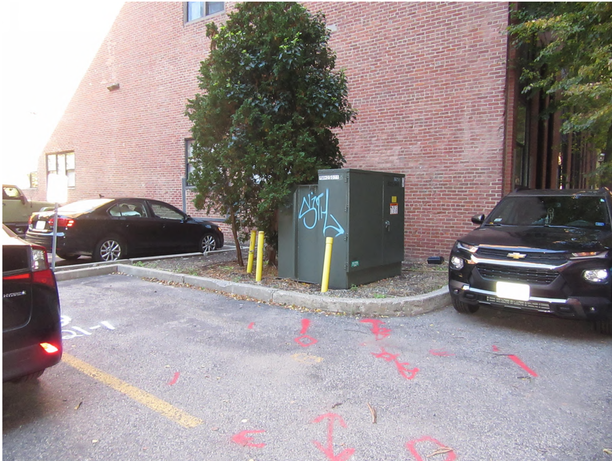
PHOTO 5 - 11 SLEEPER STREET TRANSFORMER - VIEW NORTHWEST
