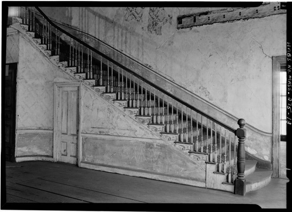
Figure 3. 1963 interior view of hall and main stair, showing remnants of partitions (upper right) installed during the building's use as a tenement (Jack E. Boucher. Historic American Building Survey – Shirley-Eustis House, MASS 13-ROX-9 , photographs. On file, Library of Congress, Washington, D.C., 1963).
