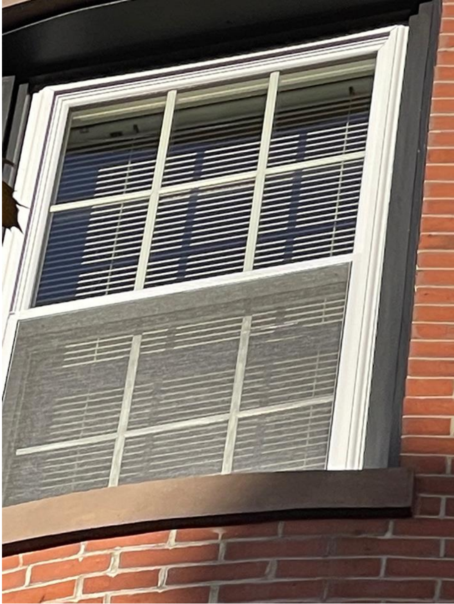
Existing window to be replaced—at the right facing street; 1 level below top floor (Photo Reference - View 2 of 2)
