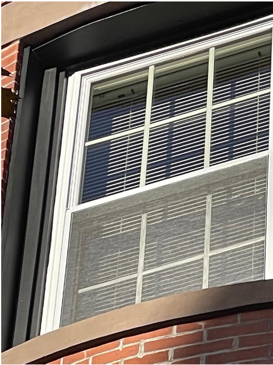
Existing window to be replaced—at the right facing street; 1 level below top floor (Photo Reference - View 1 of 2)
