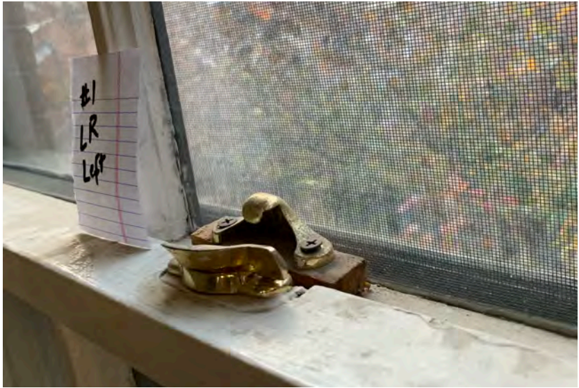
Window #1. 3rd Floor. East Side. Facing Pinckney Street. Sashes do not meet.
