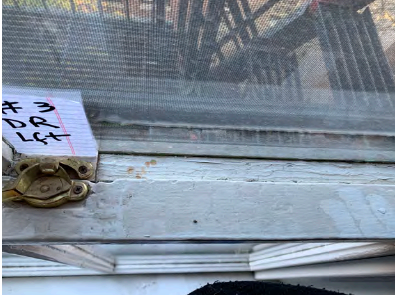
Window #3. 3rd Floor. West Side. Back side of building. Rails do not meet. Unable to lock.
