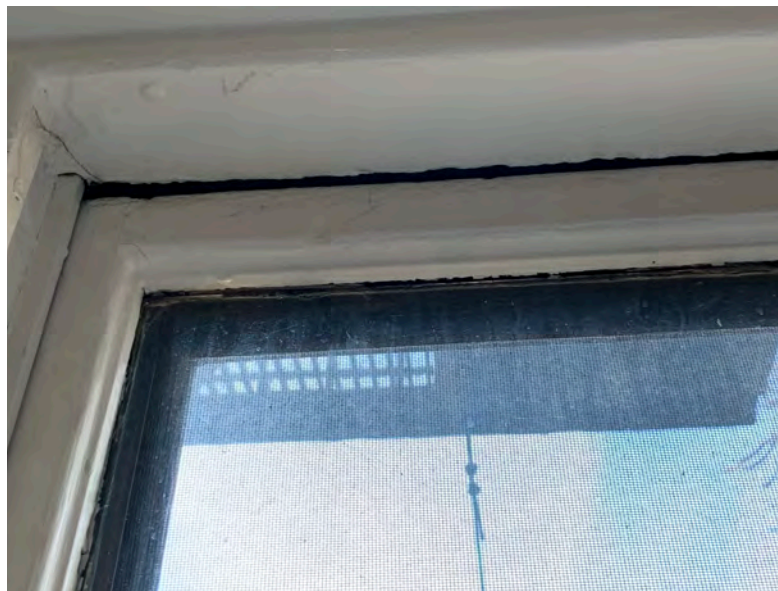
Window #4 Top Rail and Head jamb maligned, not square, sash previously modified, windows not original.
