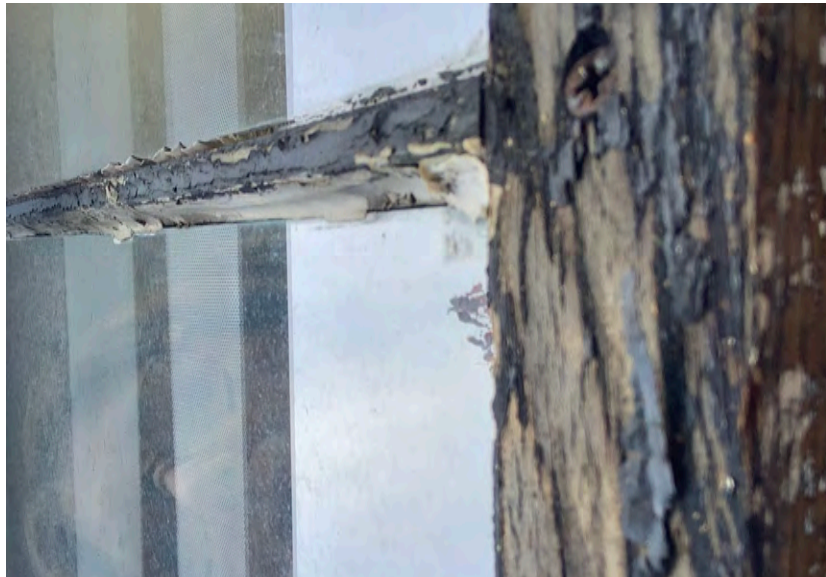
Window #2 Exterior Window Rot with screw for temporary support.
