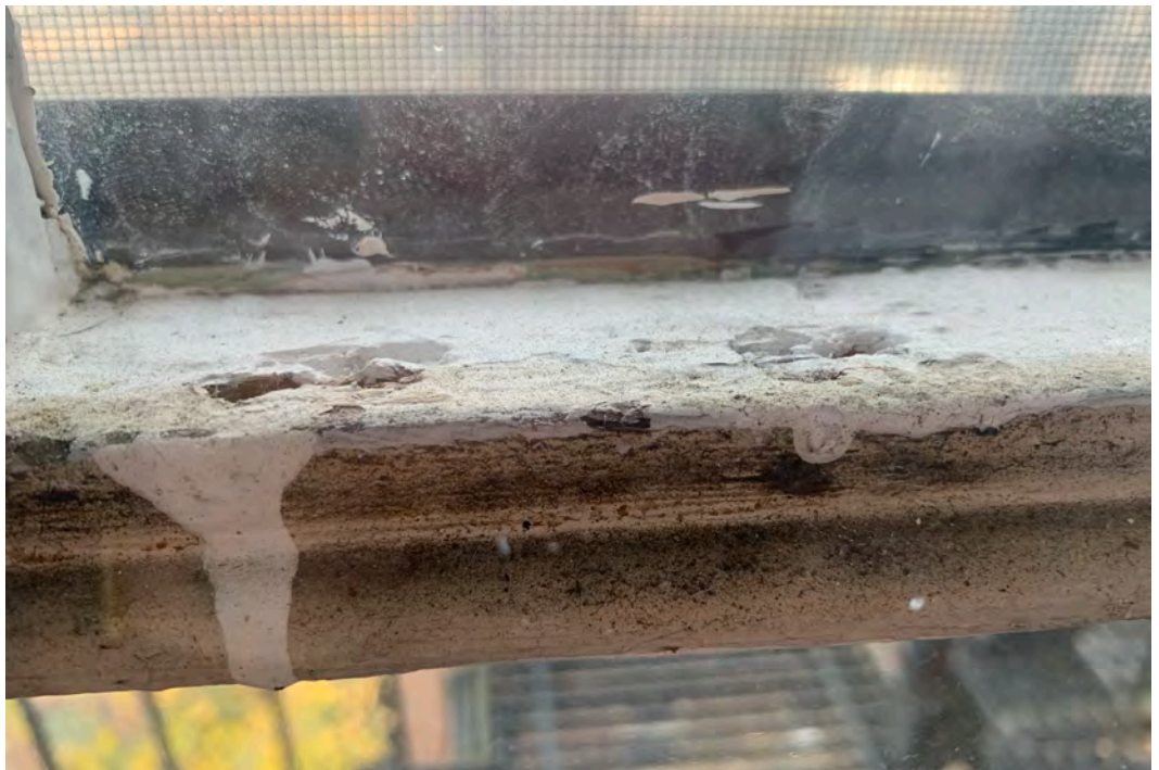
Window #8 Rot and mold
