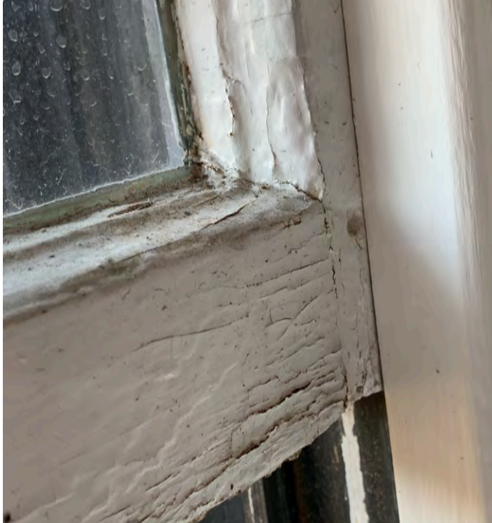
Window #4. 3rd Floor. East Side. Back side of building. Deterioration of lower sash.
