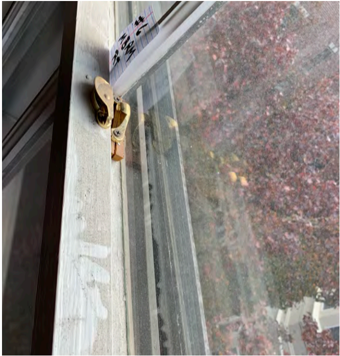
Window #5. 4th Floor. East Side. Facing Pinckney Street. Top and bottom rails do not meet. Unable to lock window.
