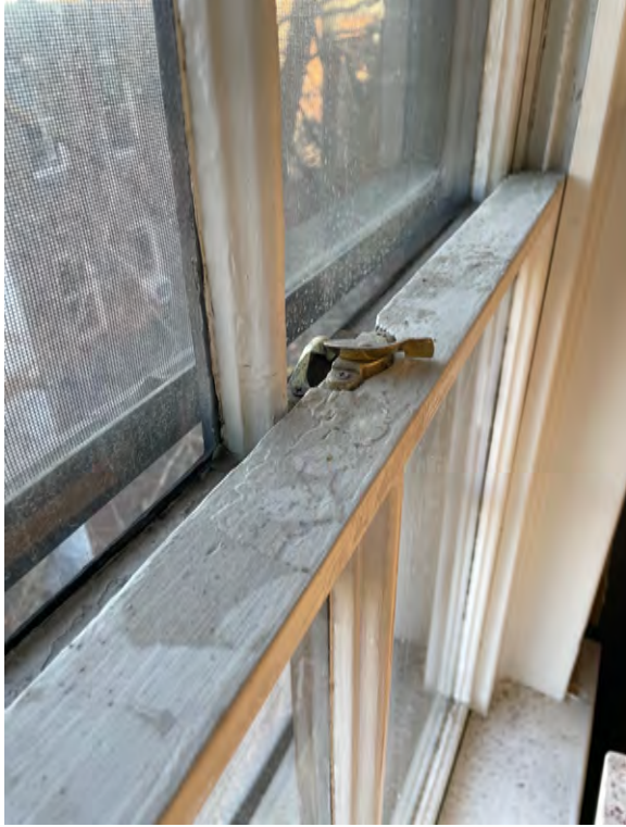
Example of existing degradation at 3 rd floor sash
