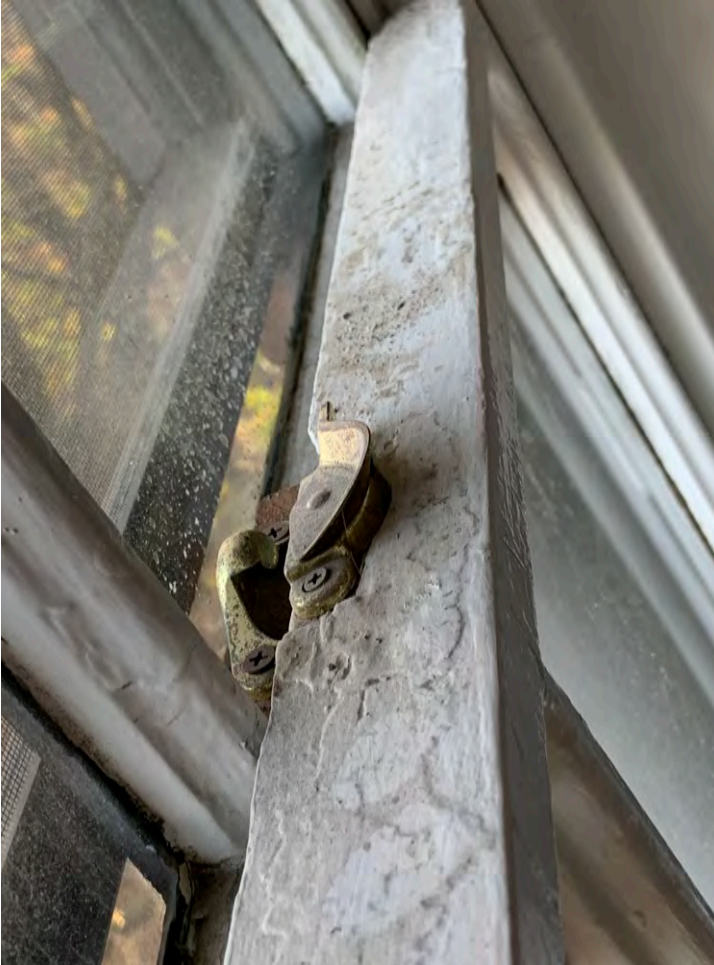
Window #3 Rails do not meet. Unable to lock.
