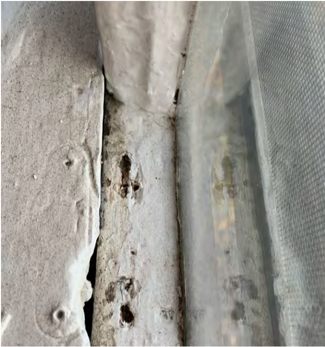
Window #8. 4th Floor. East Side. Back side of building. Lock missing due to interior rot. Poor wood integrity.
