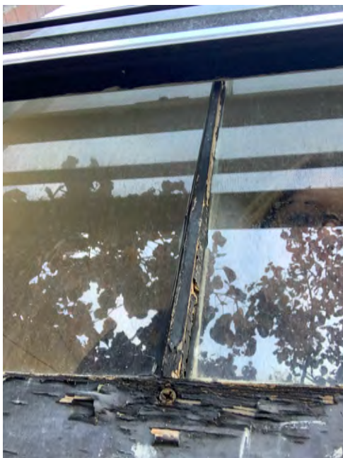
Window #2. Exterior rail rotting, held together with screw.
