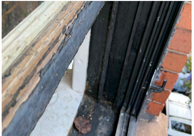
Window #2. 3rd Floor. West Side. Facing Pinckney Street. Exterior window rotting, poor integrity.
