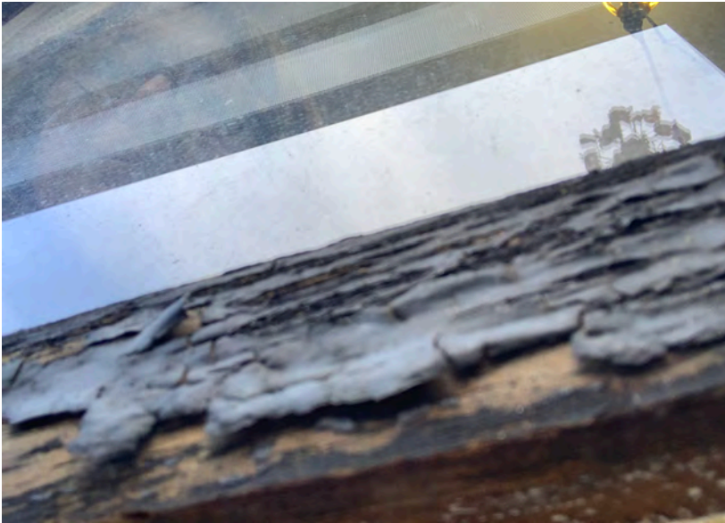
Window #2 Exterior Rot.
