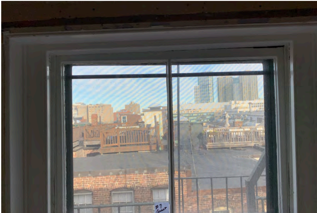
Window #7. 4th Floor. West Side. Back side of Building. Jamb is not square, rails will not fit into head jamb.
