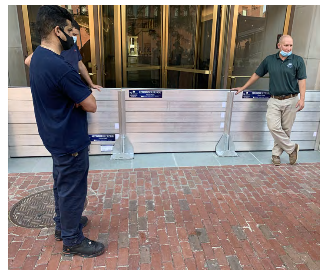
EXAMPLE FLOOD SHIELDS (INSTALLED)
