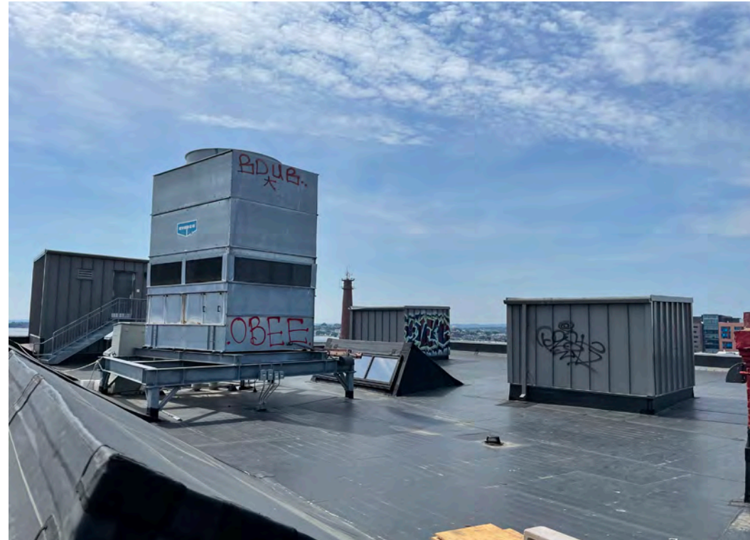
EXISTING COOLING TOWER TO REMAIN
