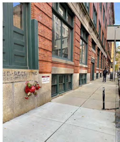
MELCHER FIRE DEPARTMENT CONNECTION
