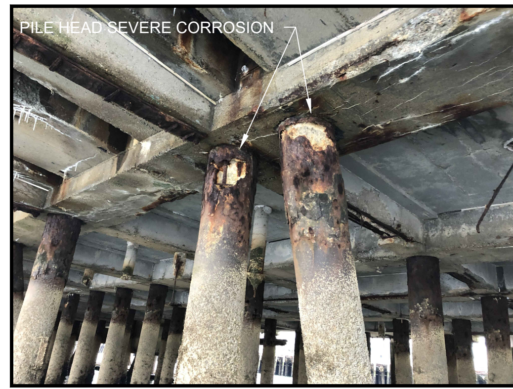
PHOTO 12 - SEVERE CORROSION AT PILE HEAD
