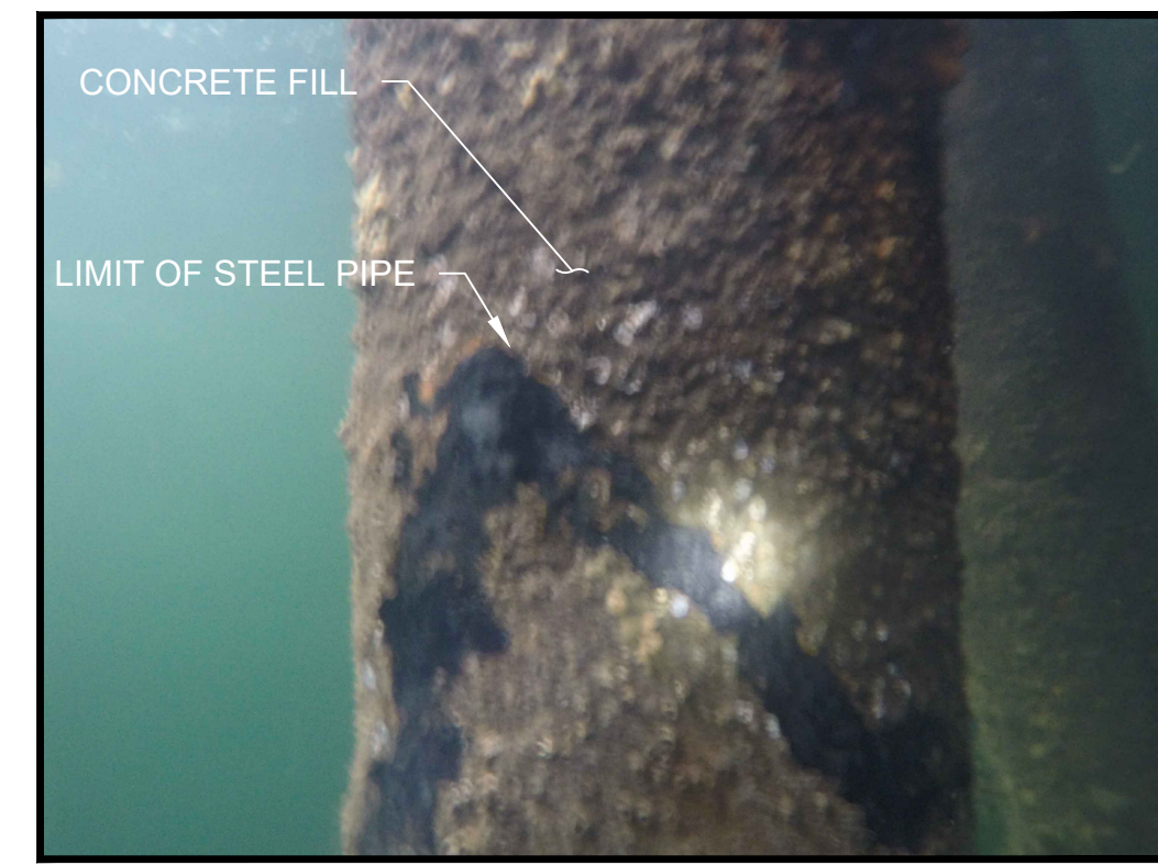
PHOTO 19 - PILE CONDITIONS UNDERWATER (TYP.)
