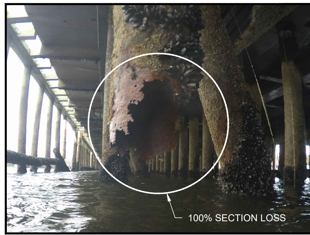
PHOTO 15 - PILE 57A 100% SECTION LOSS
