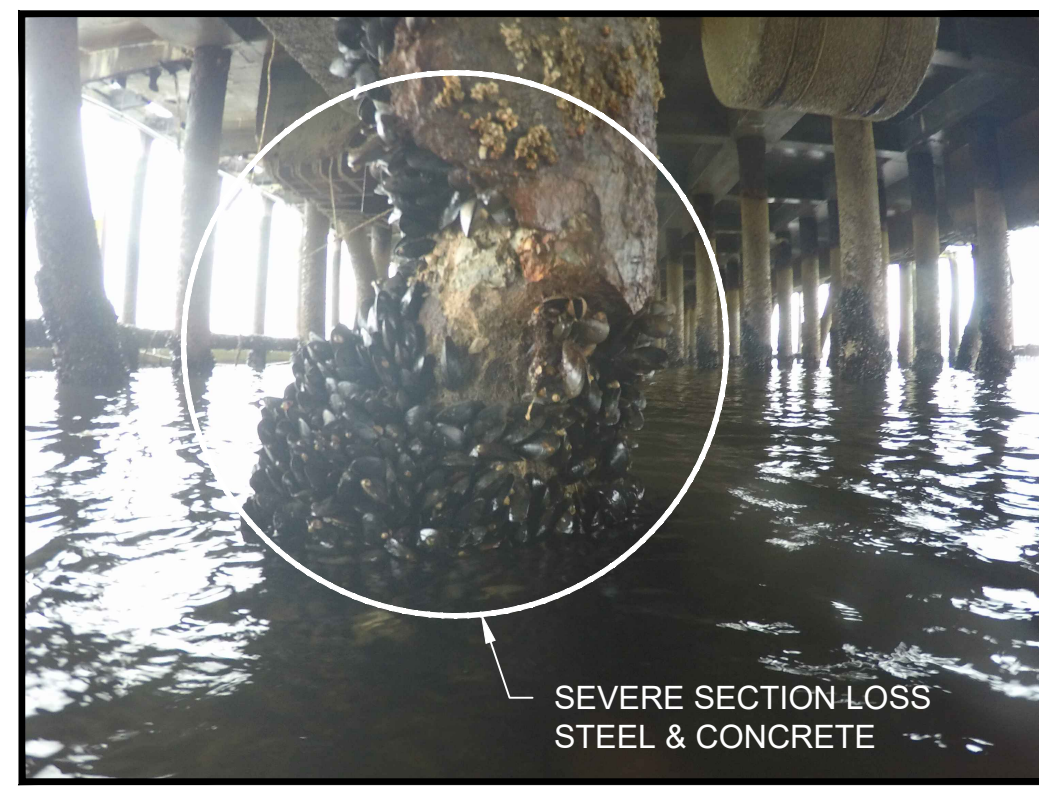
PHOTO 16 - SEVERE SECTION LOSS OF PILE
