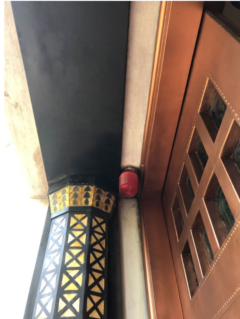
Fire department beacon to be removed
