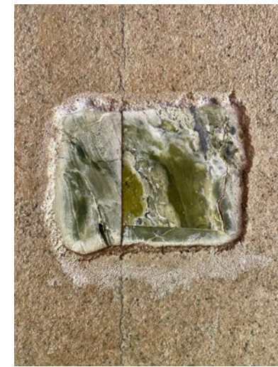
Green stone behind cementitious cladding at walls
