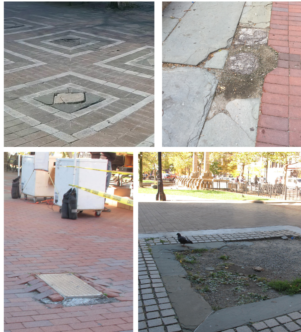
Pavements are uneven
