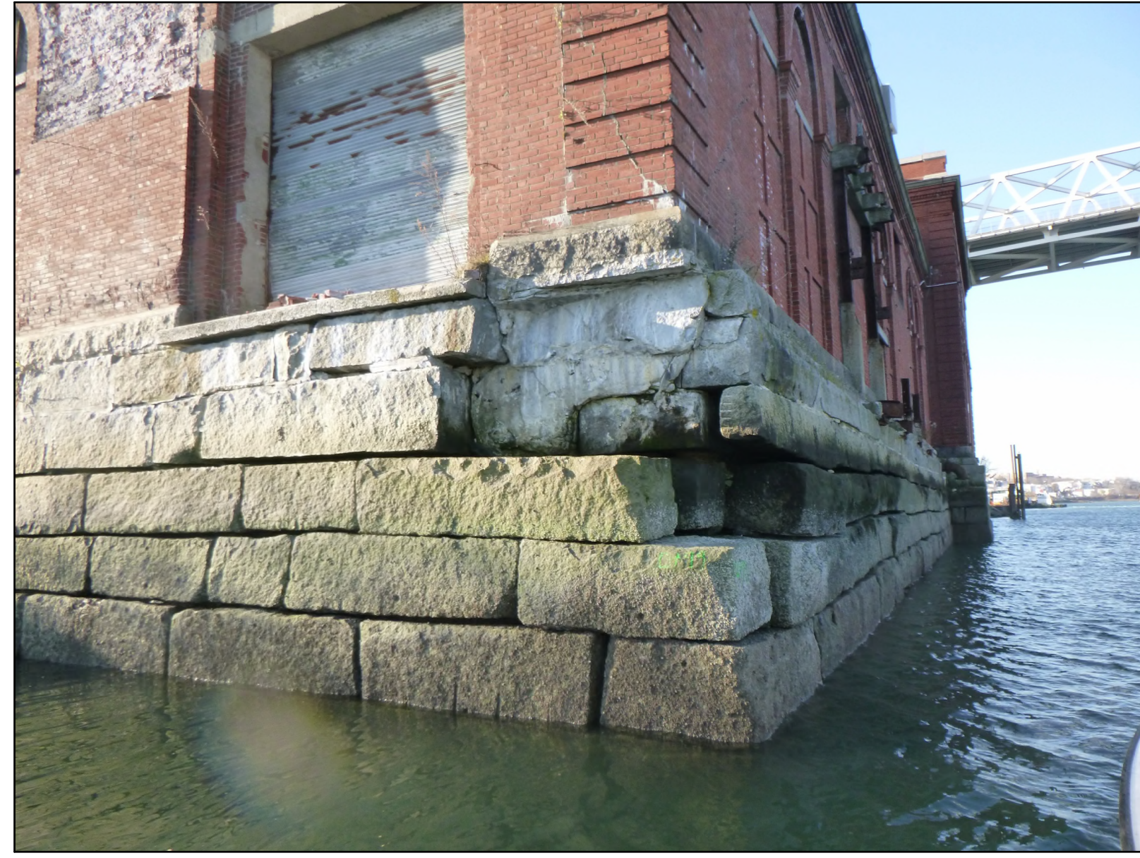
PHOTO 3: NORTHEAST CORNER OF THE BUILDING WITH VOIDS IN SEAWALL
