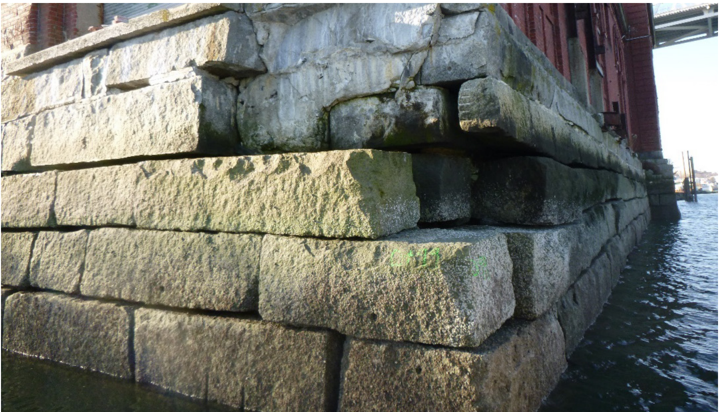
Photograph 6: Missing granite blocks within the seawall at the northeastern corner of the Pump House
