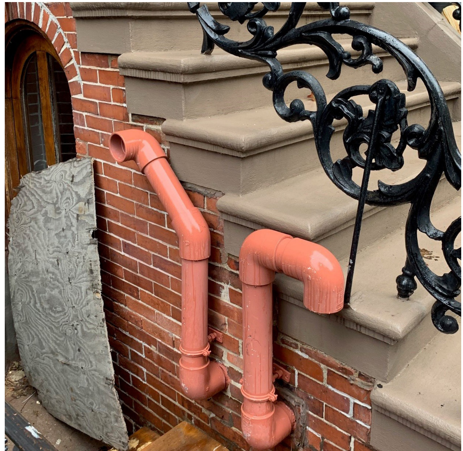
Pre-existing Condition- Left of front staircase- lower level
