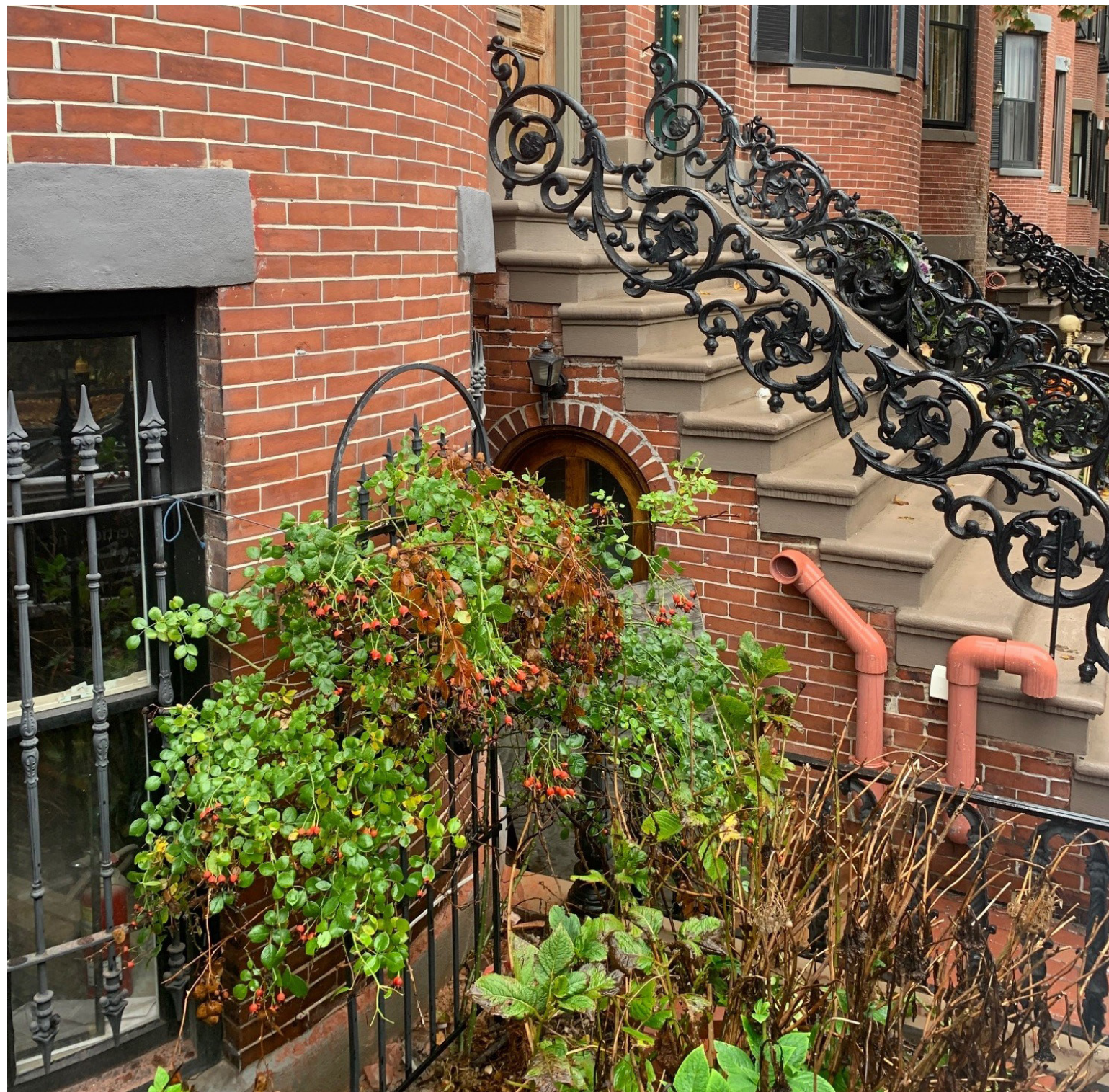
Pre-existing Condition- Left of front staircase- lower level
