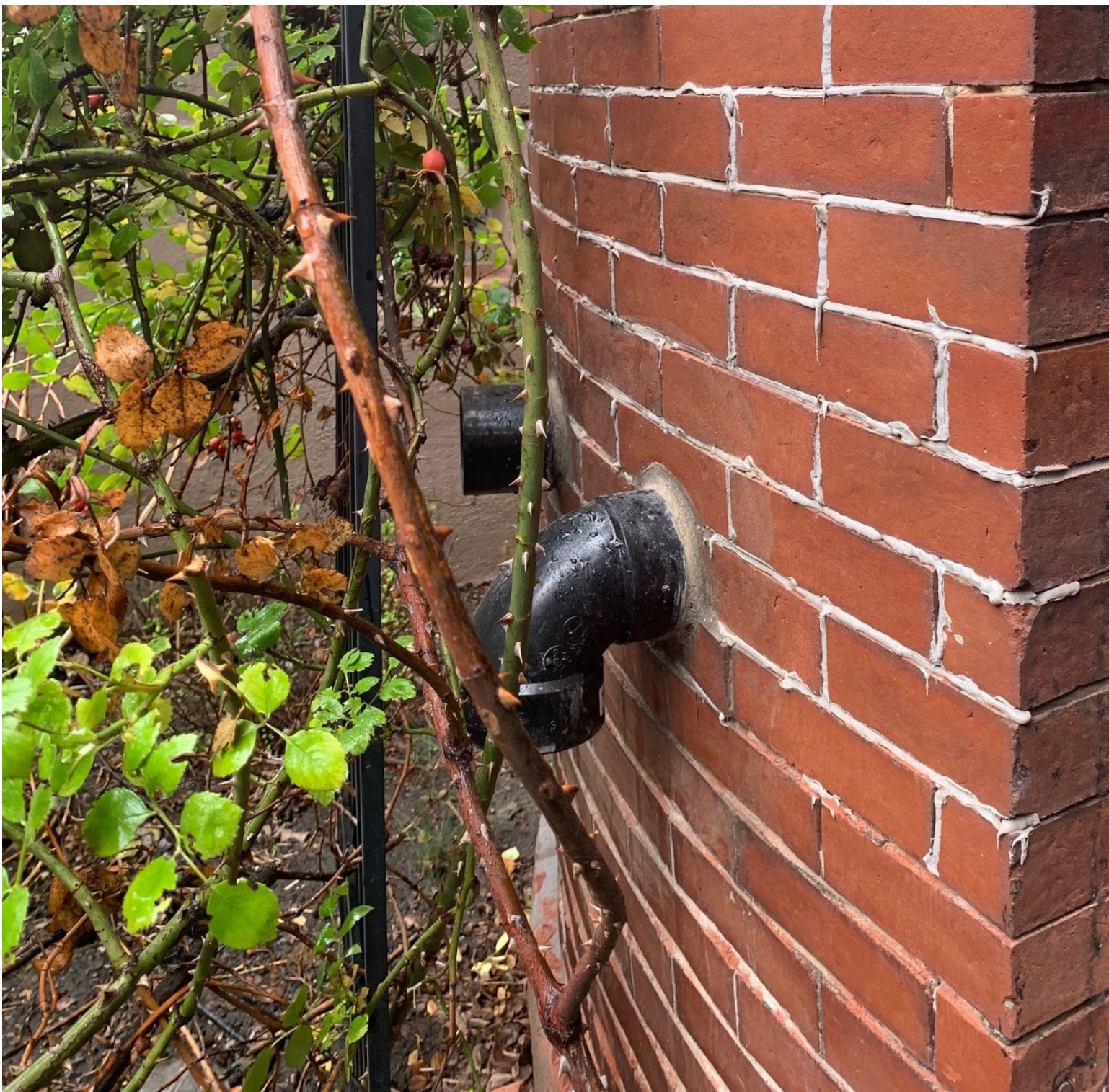
Existing Conditon- At lower level in bay
