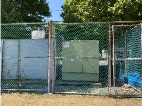
On Site Utilities
