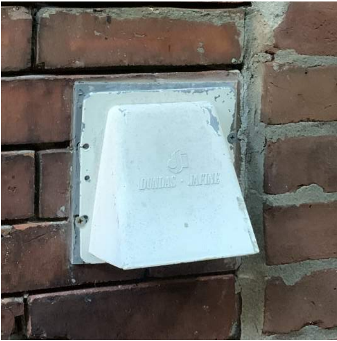
EXISTING VENT COVER AT DRYER VENT
