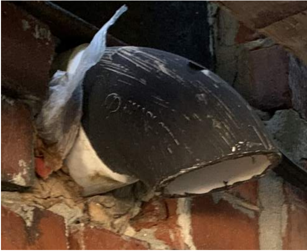
EXISTING FURNACE EXHAUST VENT (DONE BY PREVIOUS OWNER)
