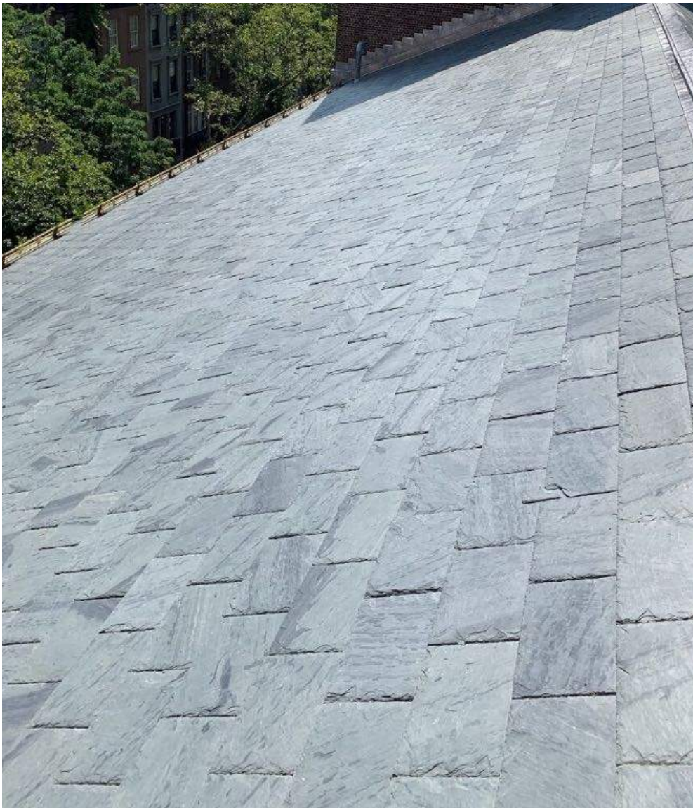
PROPOSED SLATE ROOFING (VERMONT UNFADING GRAY) SAMPLES FOR REVIEW WILL BE AVAILABLE PRIOR TO INSTALLATION
