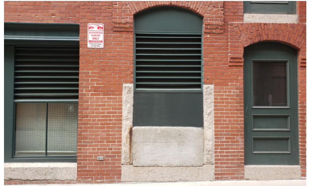
RESIDENCE INN - VENT DETAIL ON STILLINGS STREET
